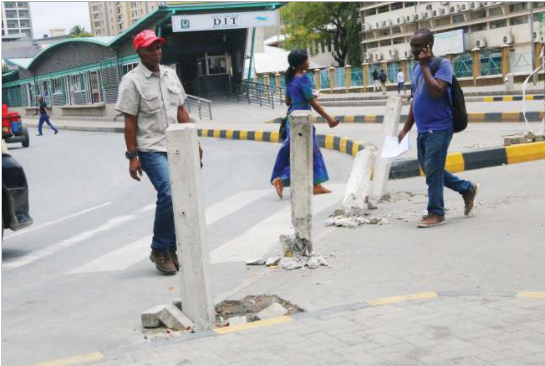
Concrete structures chiefly meant to prevent motorbike riders from disrupting flow of traffic along the Kisutu stretch of Dar es Salaam's busy Morogoro Road stand damaged and abandoned, reportedly for weeks now, as captured yesterday afternoon. Photo: Selemani Mpochi
