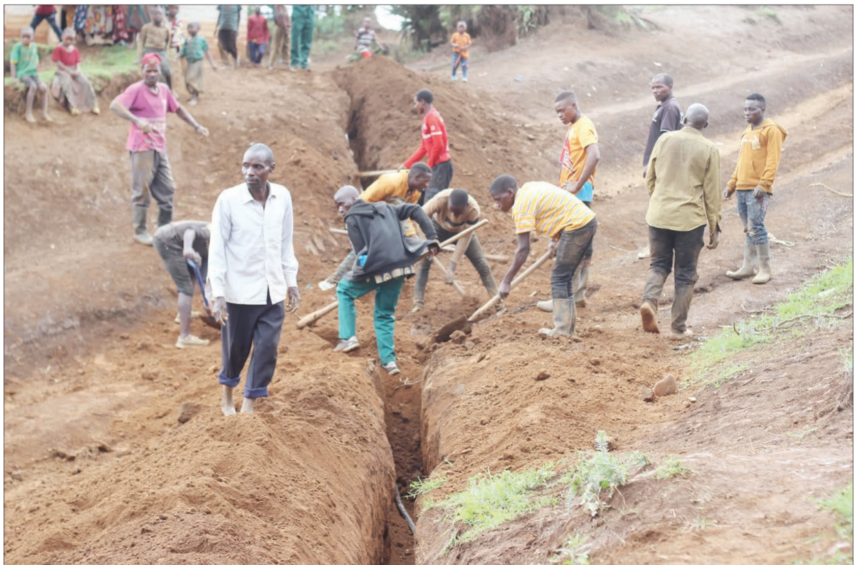
Residents of Shisyente village in Mbeya city's Masoko ward pictured late last week engaging self-help spirit in digging a trench pending the laying of a pipe for a water project being implemented by the Rural Water Supply and Sanitation Agency (Ruwasa). Photo: Correspondent Nebart Msokwa
