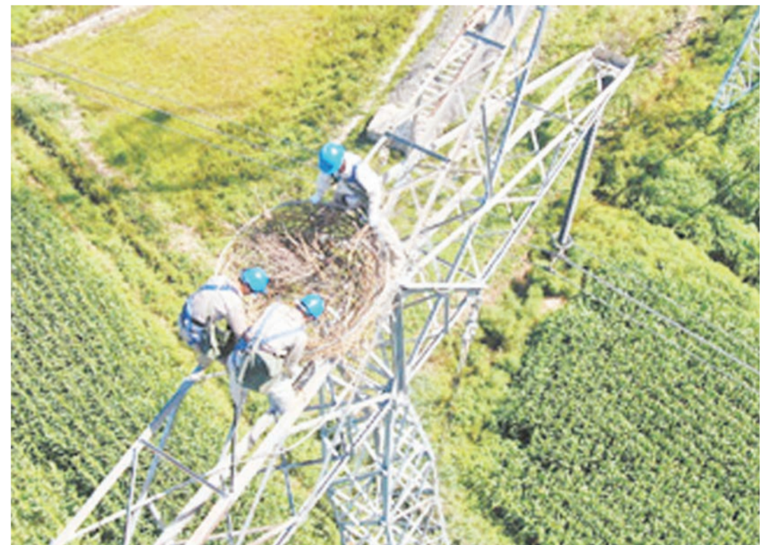
Staff members of the State Grid Corporation of China build an artificial bird nest in a safe area atop a power transmission tower. (Photo courtesy of the State Grid)
