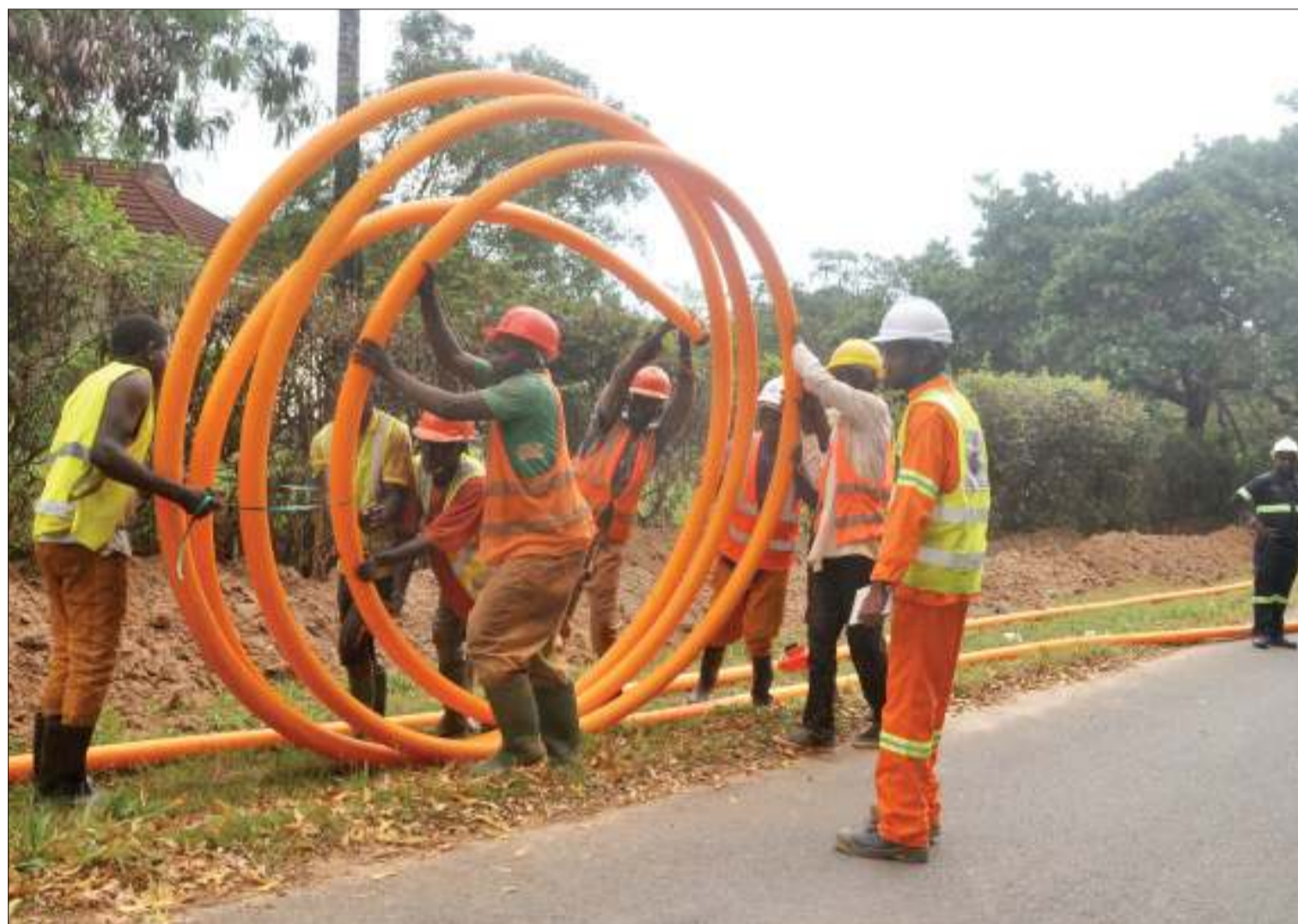
Gas Company Tanzania Ltd (GASCO) workers move to connect gas for domestic use to 85 houses in Dar es Salaam's Mikocheni suburb, including those previously lined up as minister's residences, as found earlier this week. The firm is a subsidiary of the state-owned Tanzania Petroleum Development Corporation. Photo: John Badi
