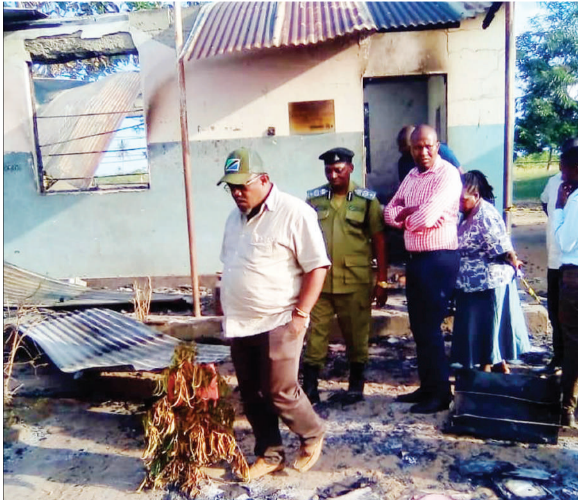
Tanga regional commissioner Adam Malima (L) leads members of the region's defence and security committee on Monday in inspecting a Marungu Secondary School building gutted by fire earlier in the day. Photo: Correspondent Hamida Kamchala
