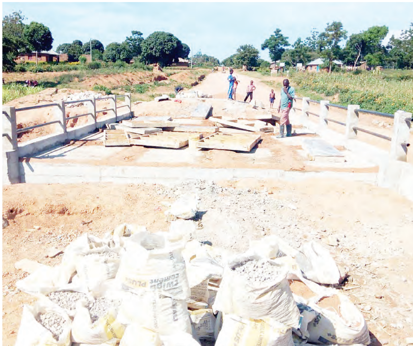
The construction of this bridge by the Tanzania Rural and Urban Roads Agency (Tarura) is nearing completion, as captured by a special correspondent earlier this week. It is a crucial link for Bulinga and Bugunda villages and other parts of Musoma Rural constituency.
