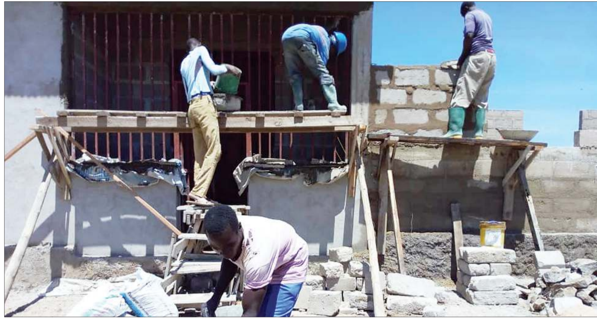
Work in progress at the construction site of a medical laboratory in the Bukima Parish of the Catholic Church in Musoma Rural as captured earlier this week, the aim being to make better health services more accessible to residents of surrounding areas. Photo: Guardian Correspondent
