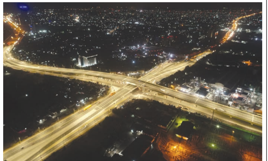
Construction of Ubungo Interchange and Associated Works under the Dar es Salaam Improvement Project (DUTP)
