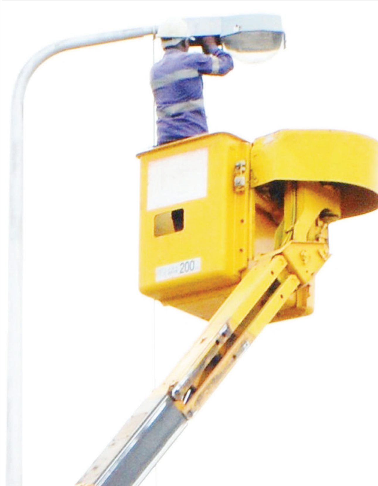
A Tanzania Electrical, Mechanical and Electronics Services Agency (TEMESA) technician repairs street lights near the Selander Bridge section of Dar es Salaam's along Ali Hassan Mwinyi Road at the weekend. Photo: Correspondent Miraji Msala
