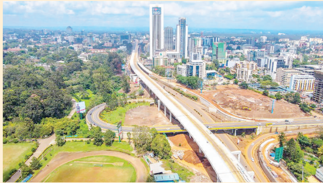
Photo taken on Dec 7, 2021, shows a section of the 27.1-km Nairobi Expressway which is being constructed by the China Road and Bridge Corporation (CRBC) in Nairobi, Kenya. [Photo/Xinhua]
