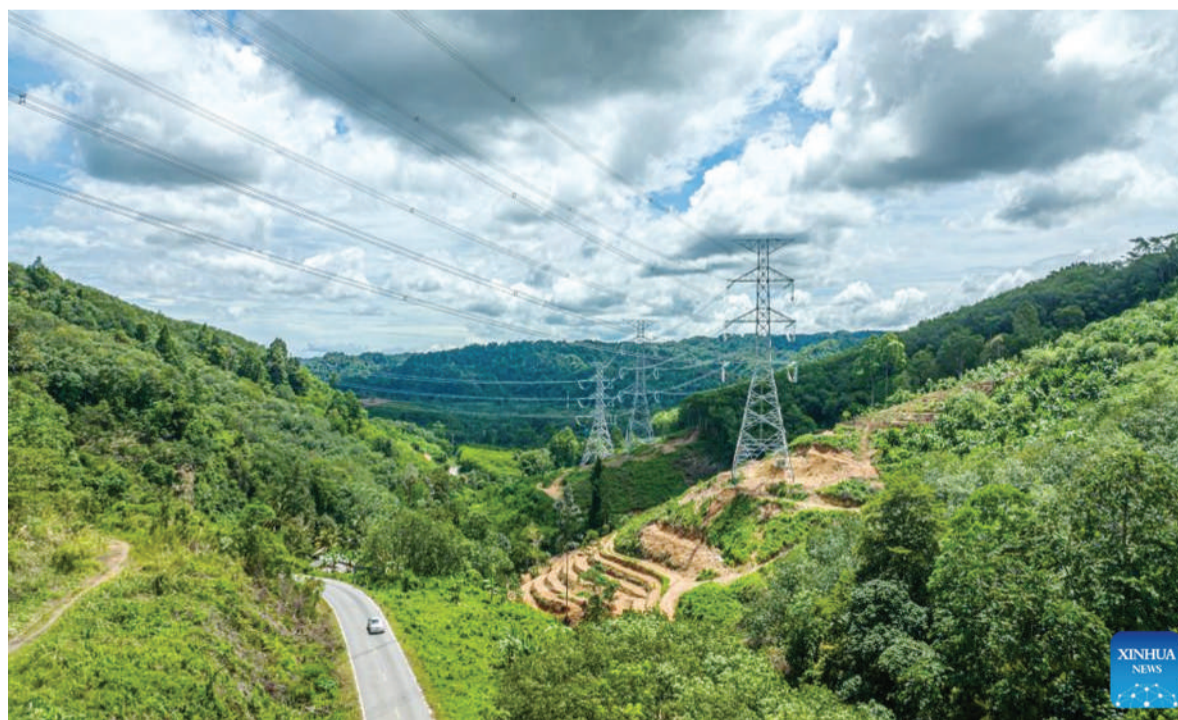
The power transmission towers in Nakhon Si Thammarat, Thailand.
