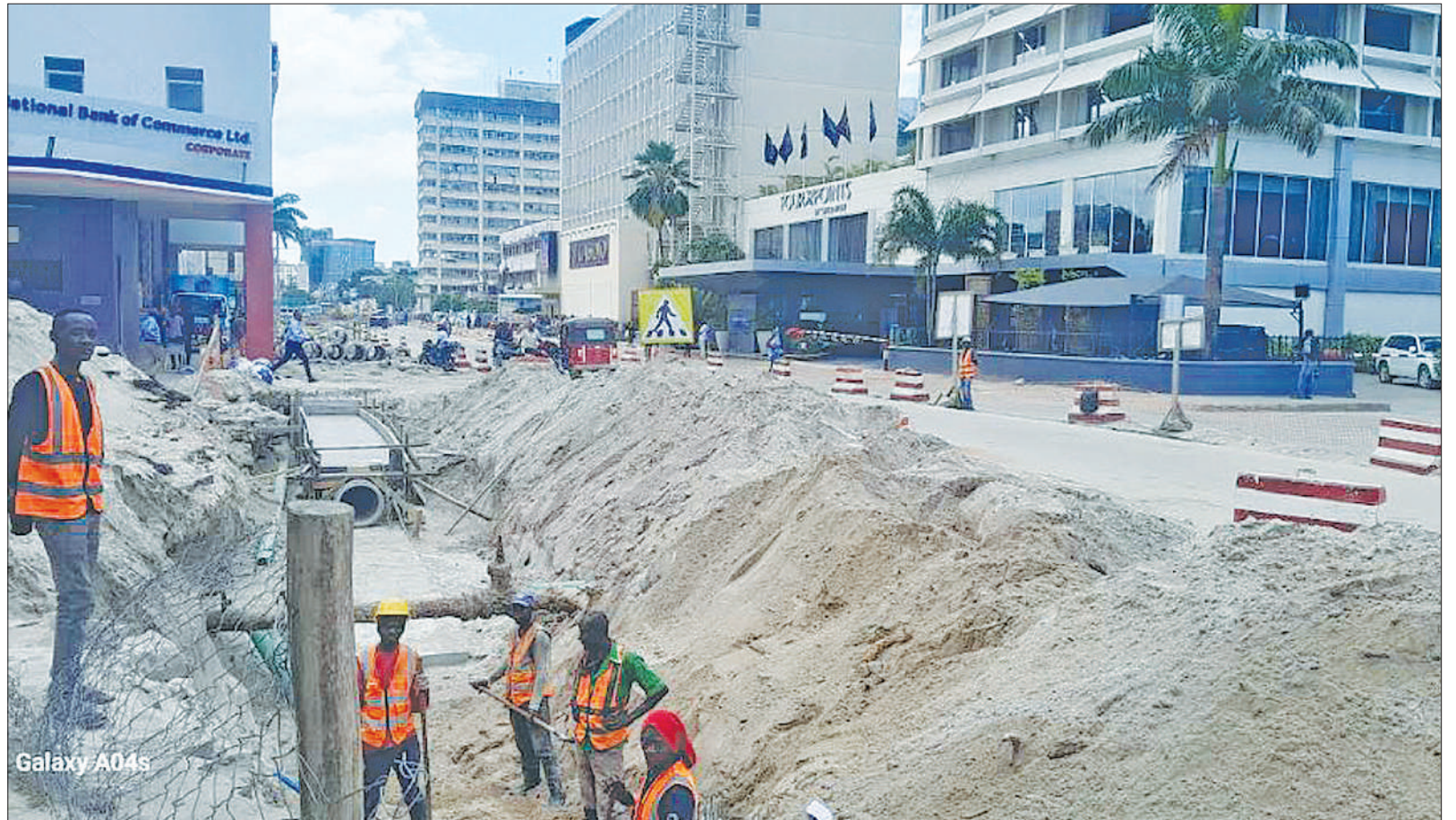
Sewage system along Azikiwe Street undergoes rehabilitation under the ongoing implementation of Dar es Salaam's ambitious rapid transit road project, as found yesterday. Photo: Correspondent Imani Nathaniel
