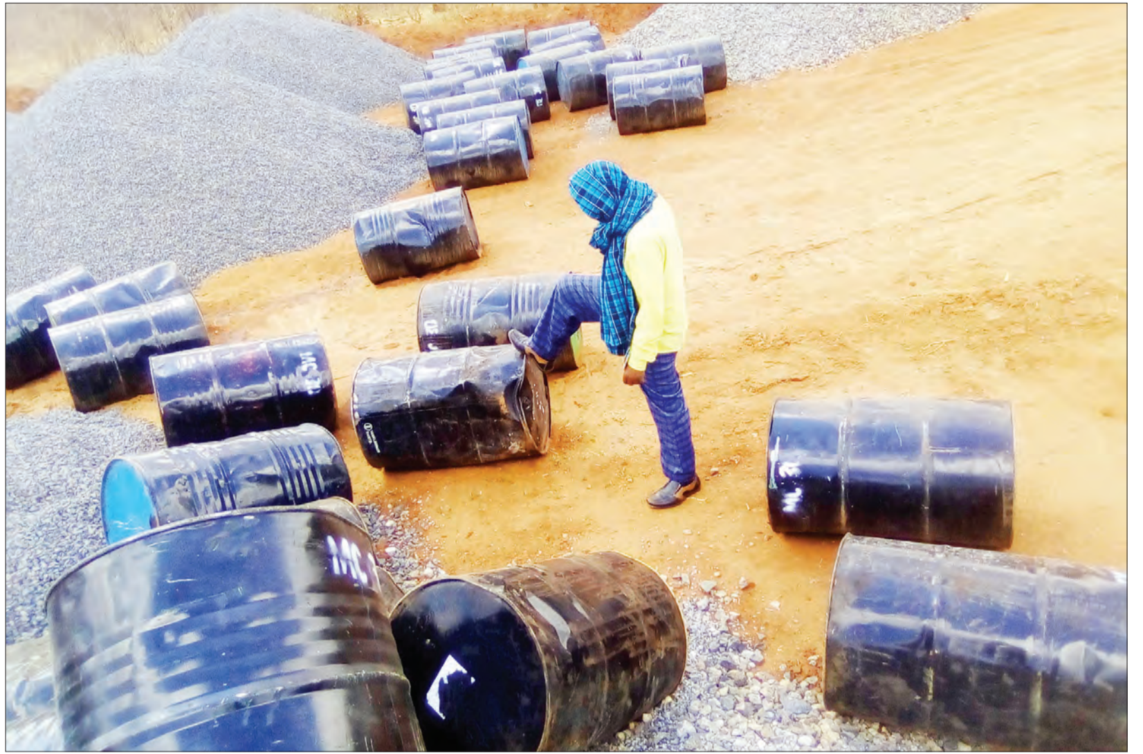
Gidewari village chairman, Baltazari Akonay shows the tarmac drums which are stored at a road construction site by TANROADS which will be used to expand mount Dabir road in Manyara region yesterday. Photo: Correspondent Jaliwason Jasson
