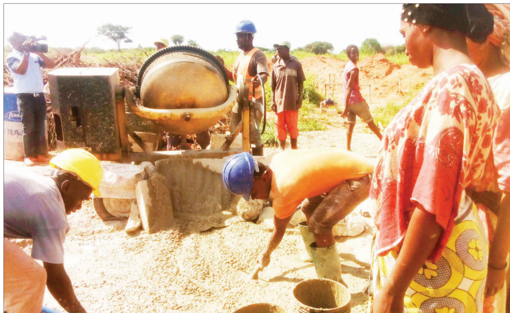
Preparations for the construction of buildings for a new Vocational Education and Training Authority (VETA) college in Mkinga District, Tanga Region, well under way yesterday. Photo: Correspondent Hamida Kamchalla
