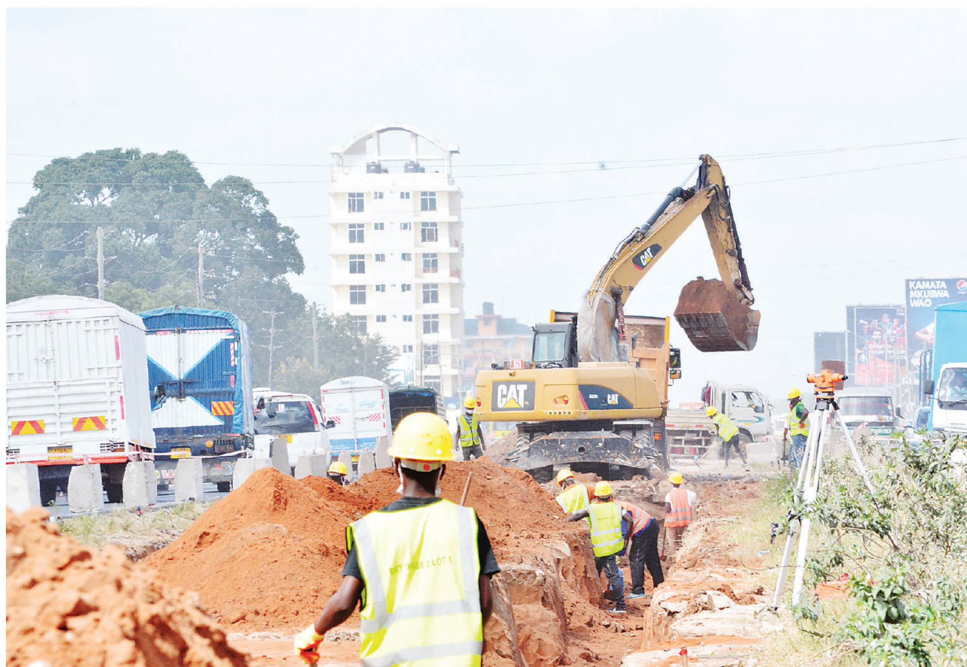
Construction of the second phase of Dar Rapid Transit infrastructure well under way along the Mbagala Kizuiani stretch of Dar es Salaam's Kilwa Road, as found yesterday. Photo: Correspondent Miraji Msala
