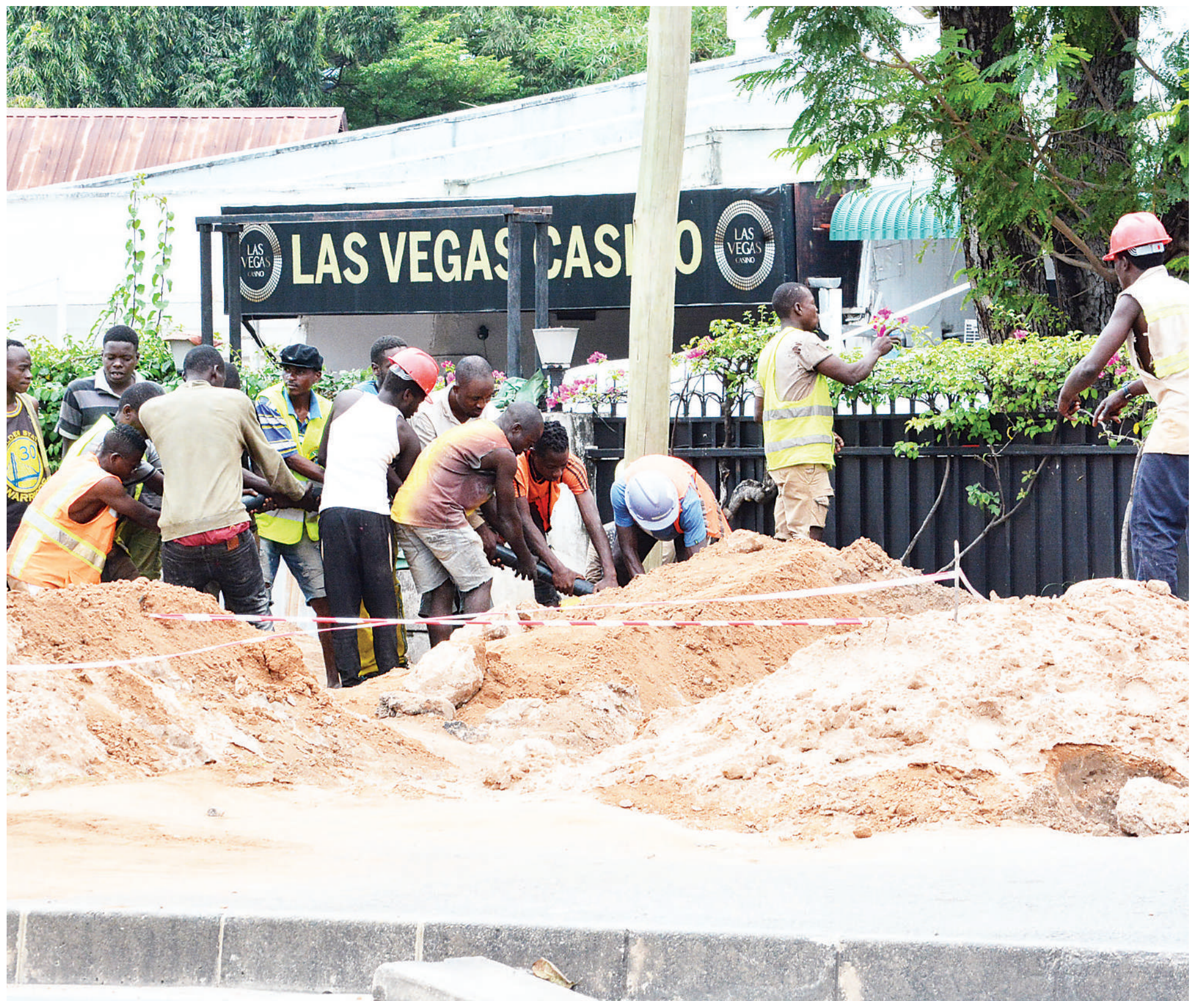
Technicians lay underground electricity cables along the Upanga East stretch of Dar es Salaam's Ali Hassan Mwinyi Road yesterday. Photo: Correspondent Miraji Msala
