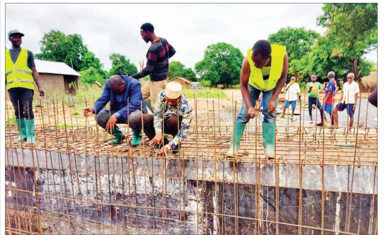
Liwale Zuberi Kuchauka (2nd-R, in cap), legislator for Liwale constituency in Lindi Region, participates in the construction of Kiyeegei bridge along the Lilombe-Liwale road at the weekend. Photo: Guardian Correspondent
