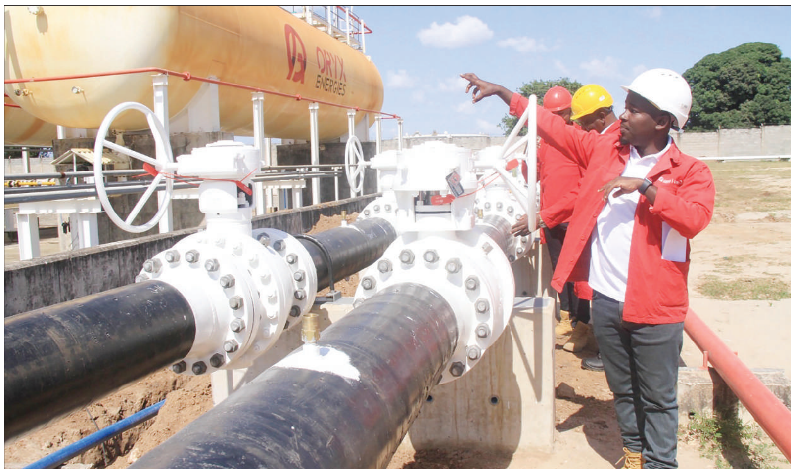
Orxy Tanzania project manager Joseph Soka pictured at the company's premises in Dar es Salaam at the weekend pointing at a pipeline which, when fully installed, will receive gas from ten countries and lead to an increase in the availability of gas for wholesale and retail sale. Photo: Guardian Correspondent
