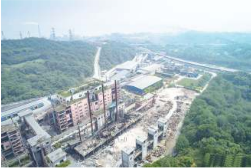
Aerial photo taken on April 30, 2018 shows the scene of the dismantling site of a chemical factory along the Yangtze River in Yichang City, central China's Hubei Province. Since 2017, Yichang has carried out a series of projects to cut pollution and upgrade the chemical industry to protect the ecological environment along the Yangtze River. (Xinhua)
