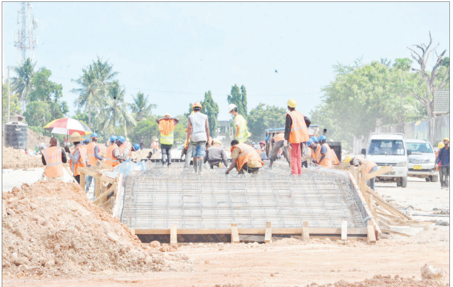
Rehabilitation of Dar es Salaam Rapid Transport bus stand under way, as captured yesterday. Photo: Correspondent Miraji Msala
