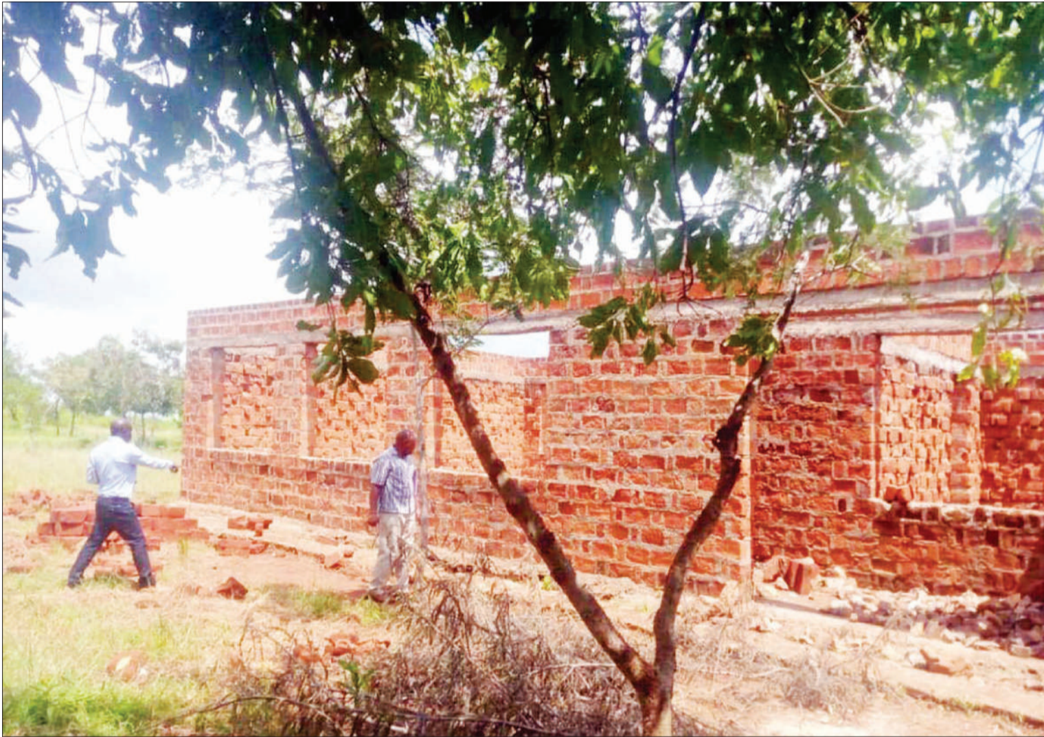
This is one of several classroom buildings undergoing construction, as found earlier this week at Mabuimerafuru Secondary School in the Musoma Rural constituency on a self-help basis, chiefly with a view to accommodating newly enrolled Form I students sometime later this year. Photo: Guardian Correspondent
