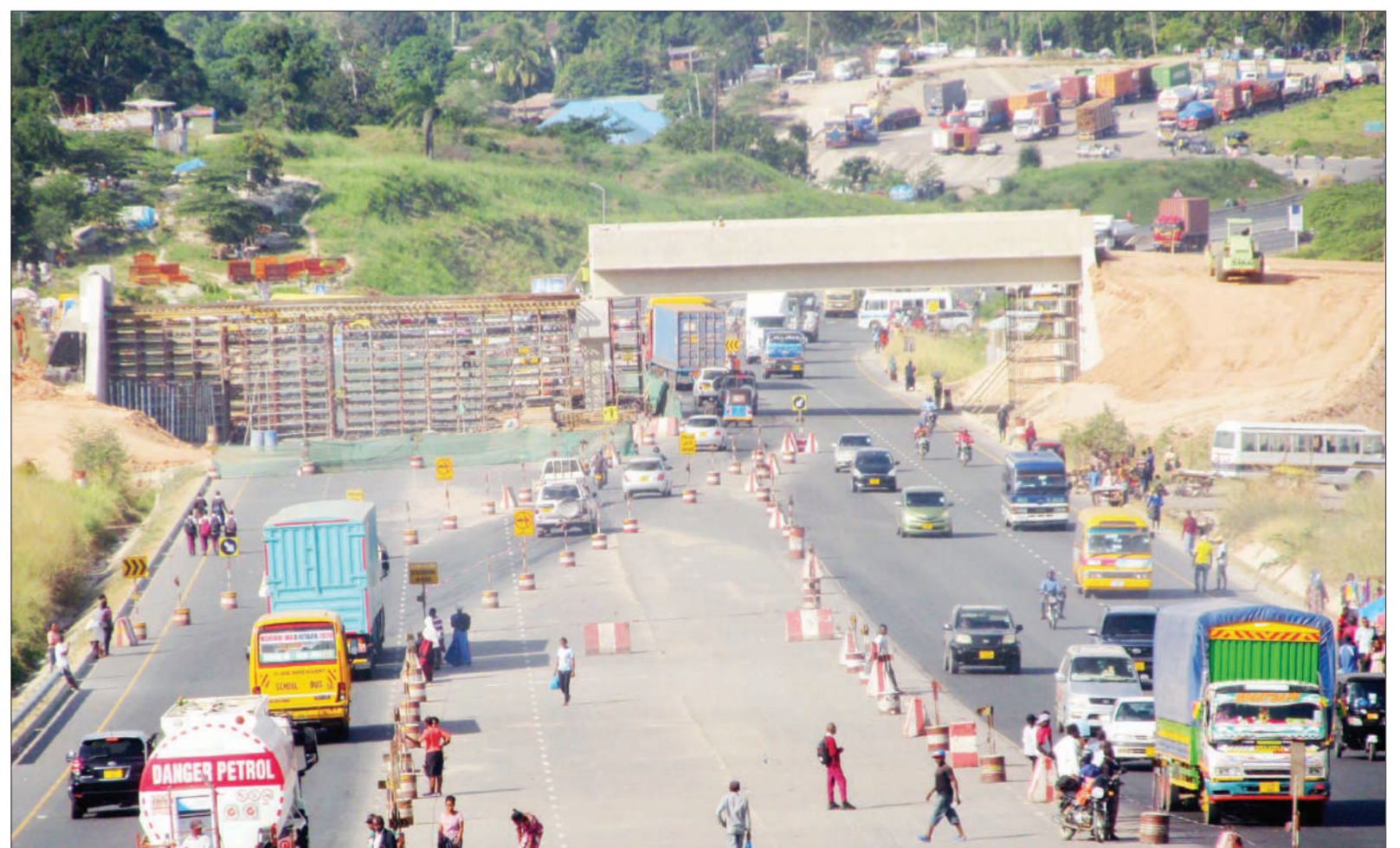
Mbezi Mwisho flyover project in the outskirts of Dar es Salaam is one of the many infrastructure projects that the sixth phase government is executing to ease traffic congestion. Photo: Correspondent Sabato Kasika
