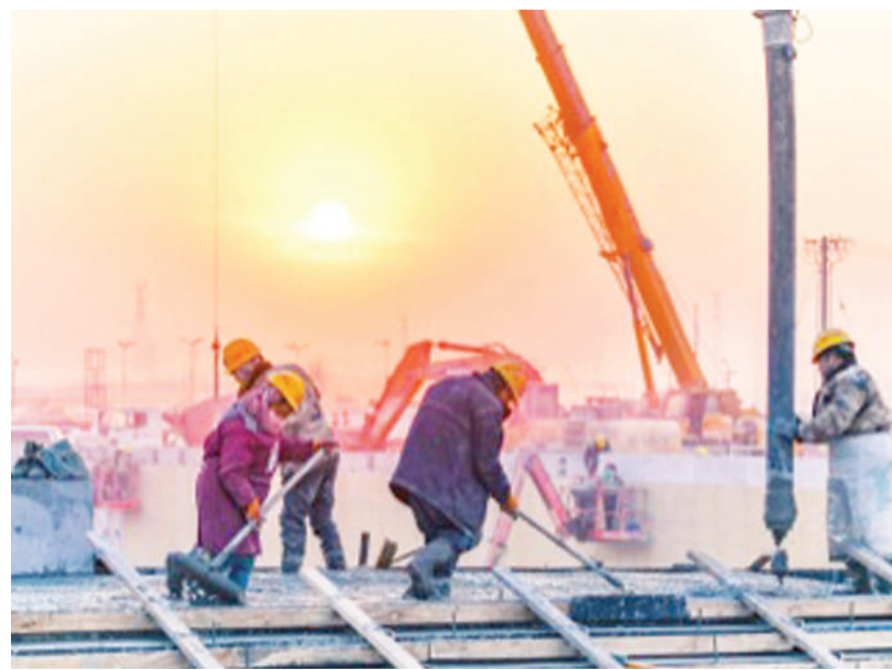
Photo taken on Dec. 19, 2020, shows construction workers busy with the final construction of the west square of the Xiong'an Railway Station in Xiong'an New Area, north China's Hebei province.
