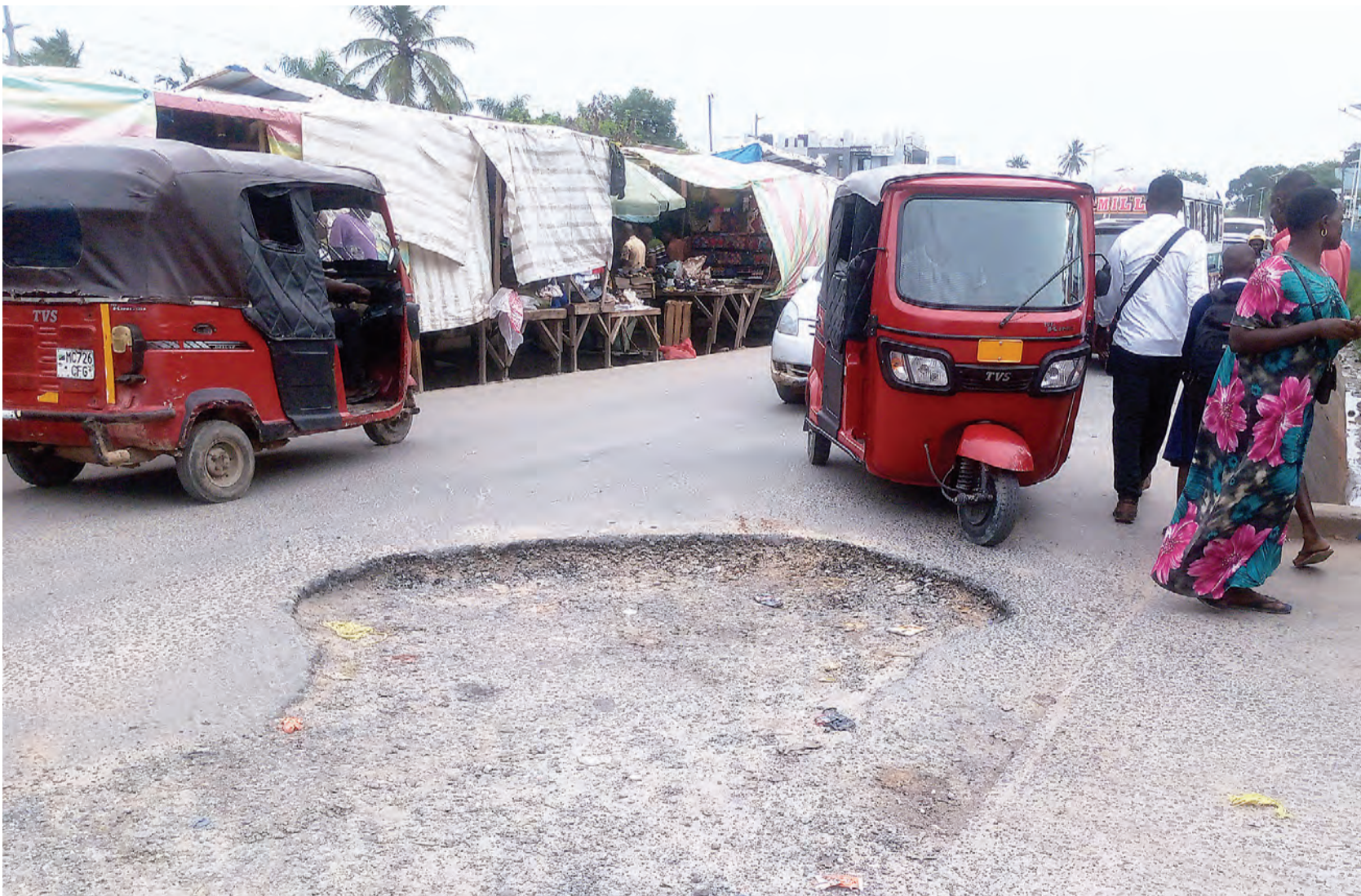
With such a gaping pothole in place, what road would be 'friendly' enough to vehicular traffic? Yet, this is the state this Mbezi Mwisho section of Malamba Mawili Road in suburban Dar es Salaam has been in reportedly for over three months now. Correspondent Sabato Kasika captured the scene yesterday.
