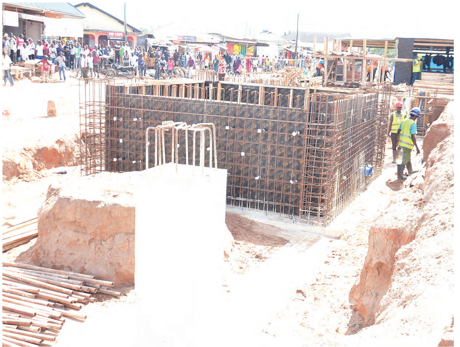
Construction of an apparently unique-looking sewage and rainwater drainage system draws crowds at a point in Dar es Salaam's Buguruni suburb on Thursday. Photo: Correspondent Jumanne Juma
