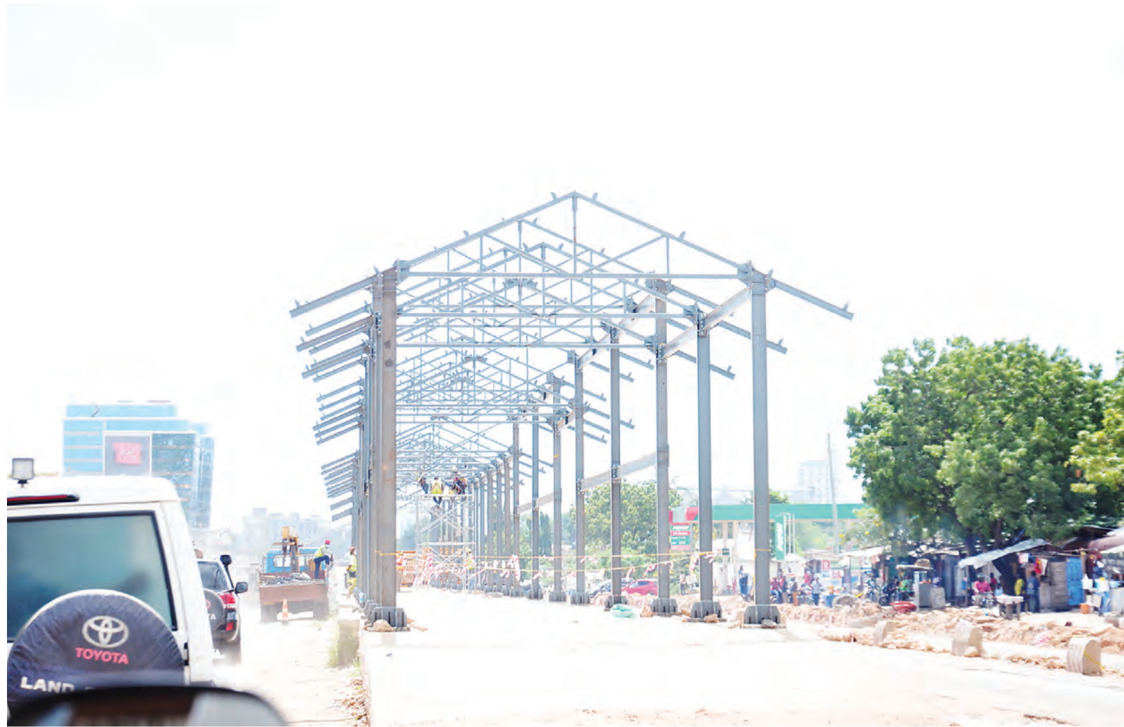
A view of a Dar es Salaam rapid bus transit (BRT) project bus stop still undergoing construction - at the Sido section Nyerere Road - as captured on Thursday. Photo: Correspondent Jumanne Juma
