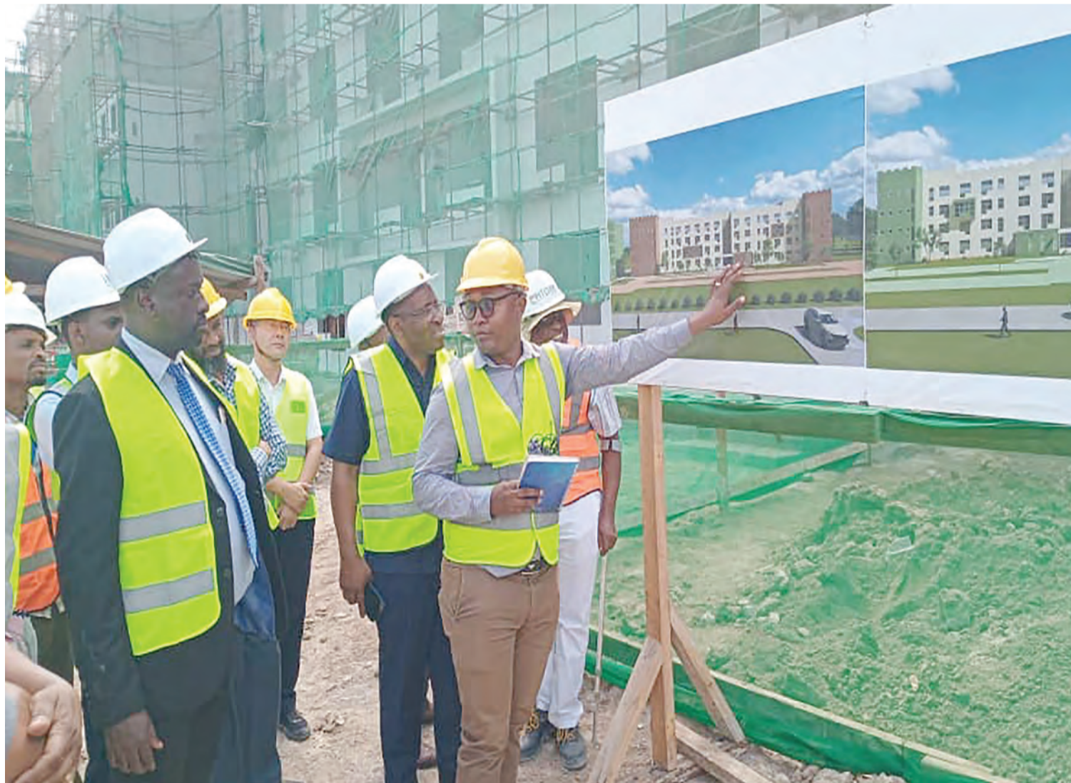
Dr. Fredrick Salukele (L), Director of Vocational Training at the Ministry of Education, Science and Technology, listens to Saimon Moshi, the Epitome site engineer, as he explains a building project at NIT supported by the World Bank's Eastrip project. Photo: Correspondent Prosper Makene
