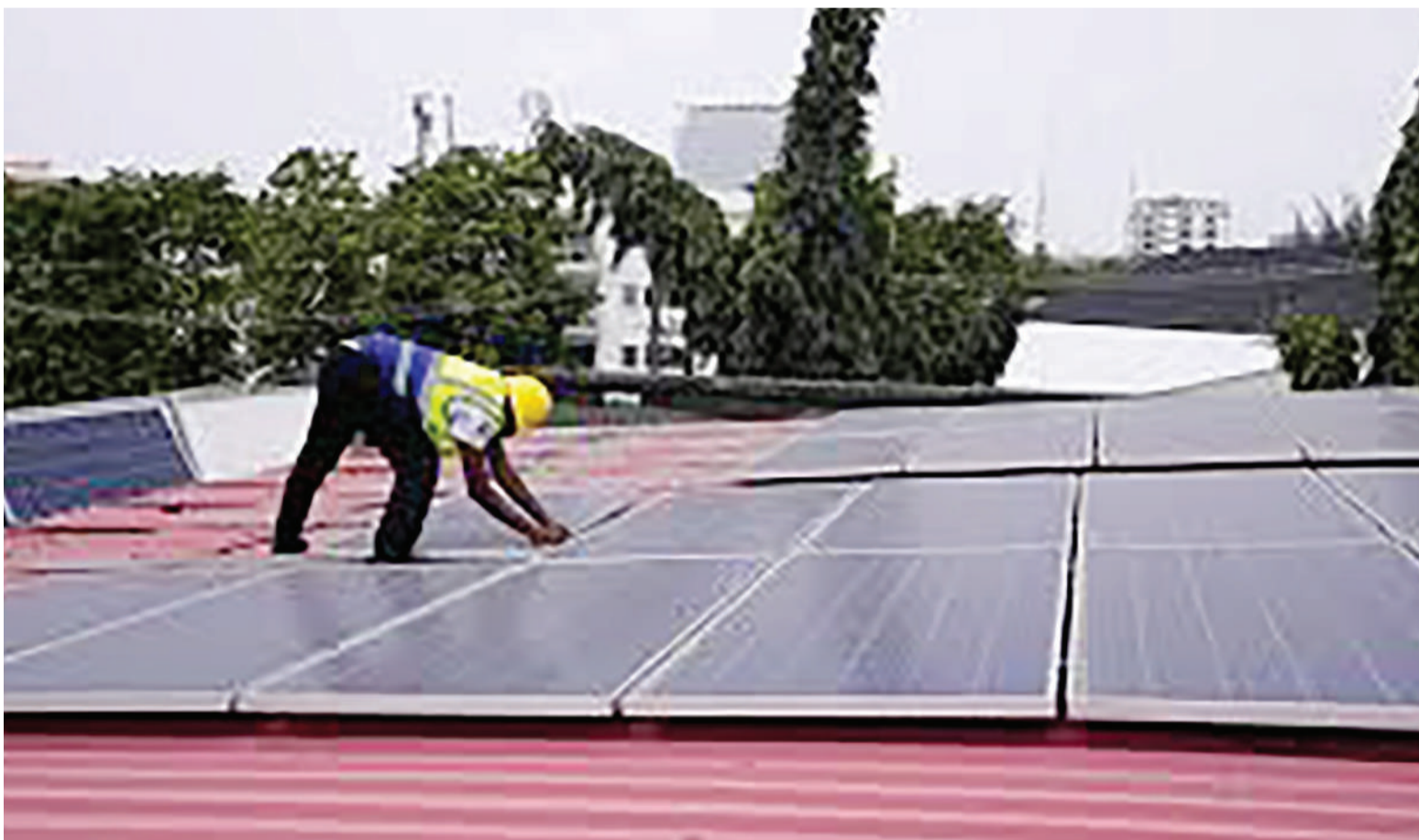
Oladapo Adekunle, an engineer with Rensource Energy, installs solar panels on a roof of a house in Lagos, Nigeria.
