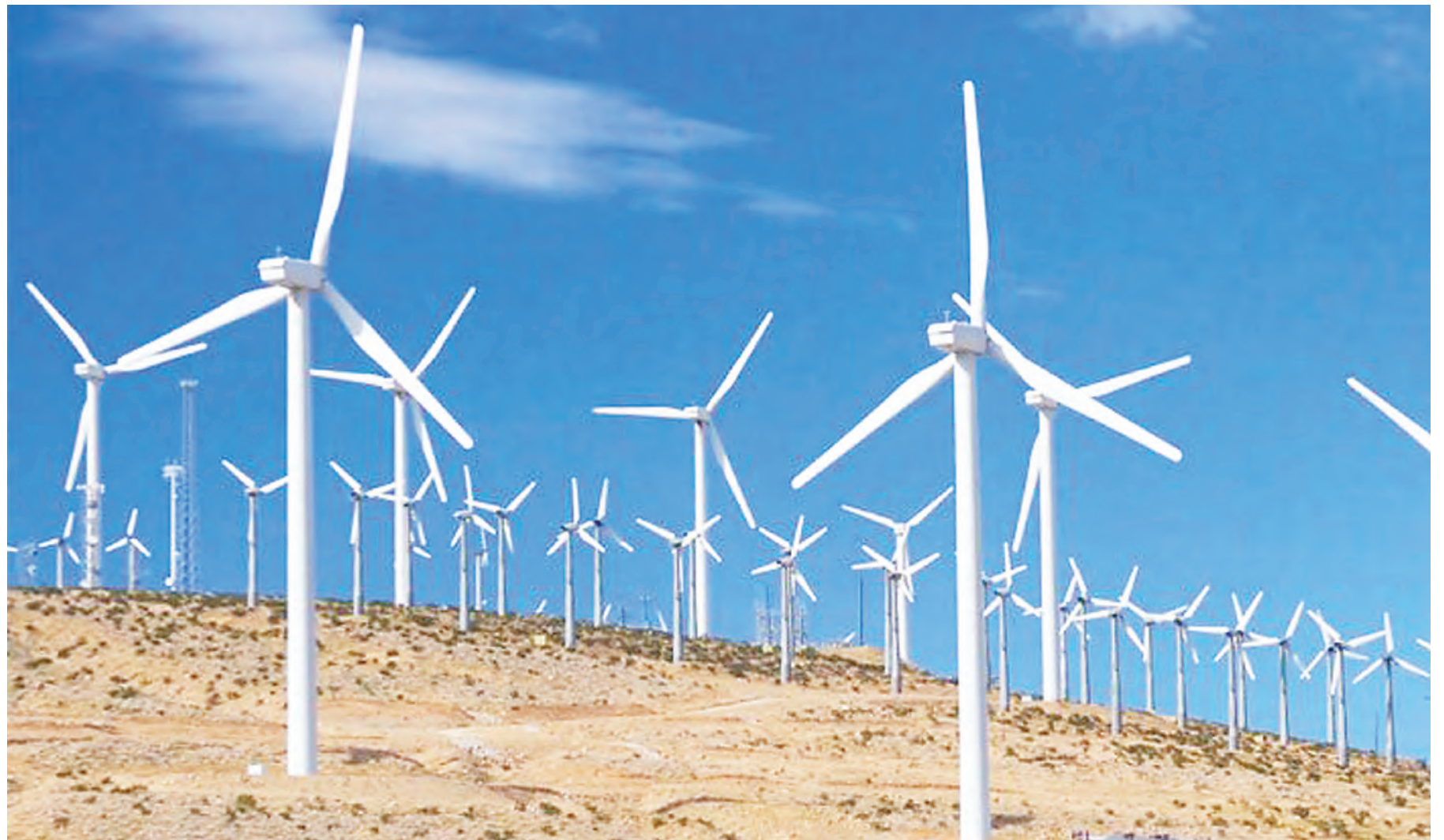
A wind power plant in Singida Region
