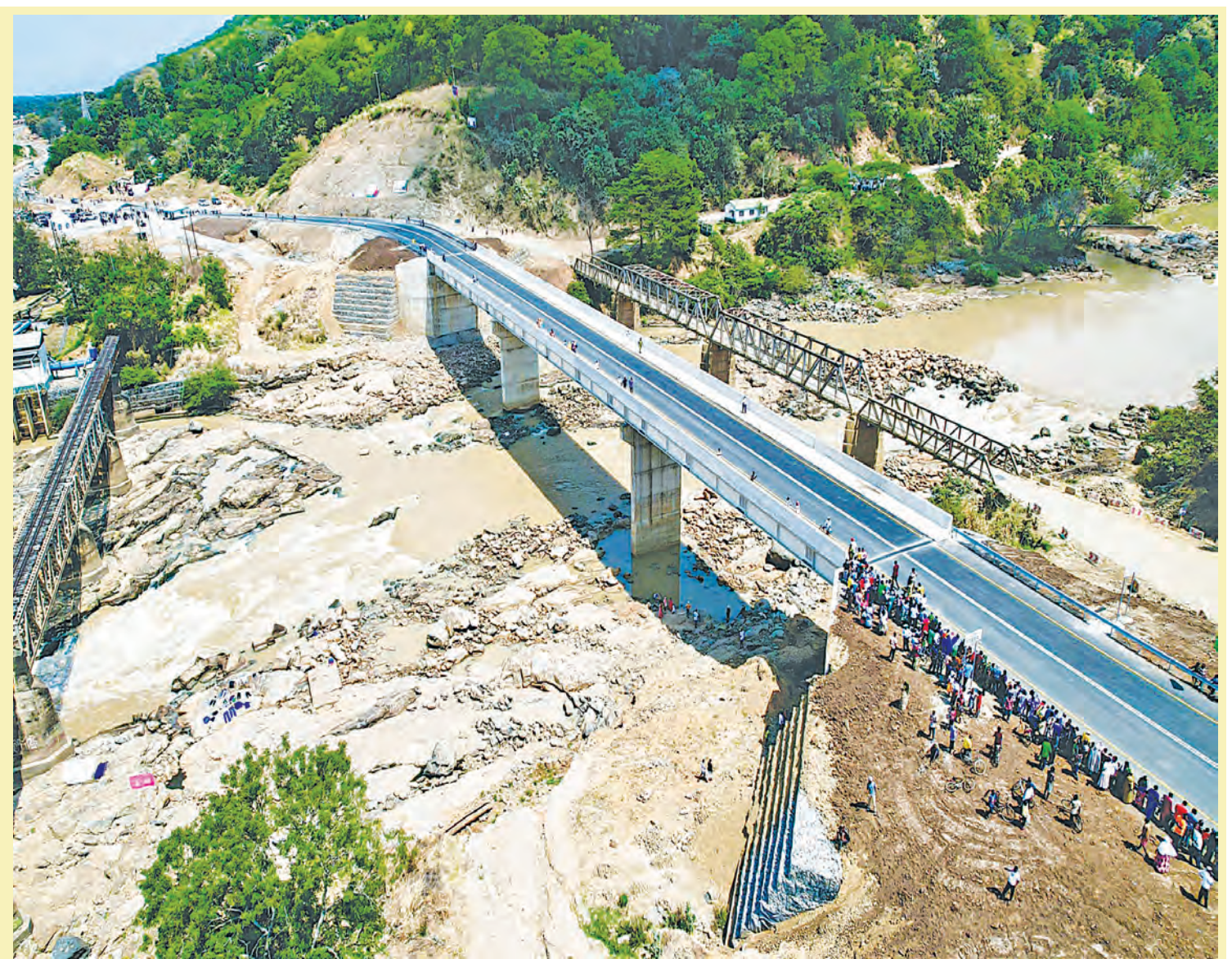
This is an aerial view of the 133-meter-long Ruaha Mkuu Bridge, as captured at the weekend. It is a strategic section of the 66.9-km Kidatu-Ifakara road, whose construction to tarmac level was completed recently and which President Samia Suluhu officially opened on Sunday as part of her week-long working tour of Morogoro Region. Photo courtesy of Works ministry
