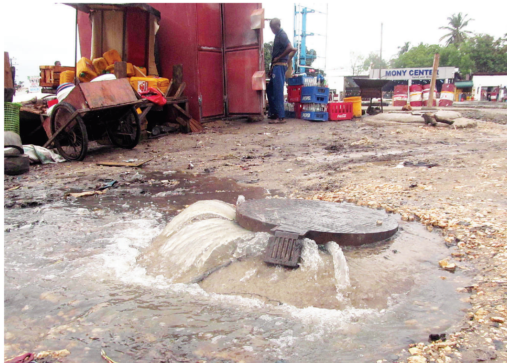
This defective sewage chamber right in the middle of the road near the main mixed-goods market in Dar es Salaam's Mwenge suburb has been intermittently spewing stinking effluent for months now, clearly endangering public health. Correspondent Sabato Kasika's roving camera captured the scene yesterday.
