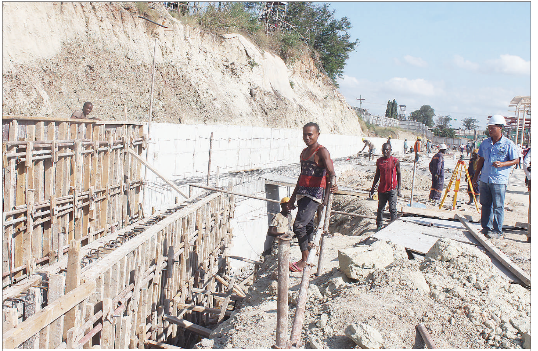
Work at the site of suburban Dar es Salaam's long-stalled Mbezi Luis bus terminal project in progress, as found earlier this week. Photo: Correspondent Jumanne Juma
