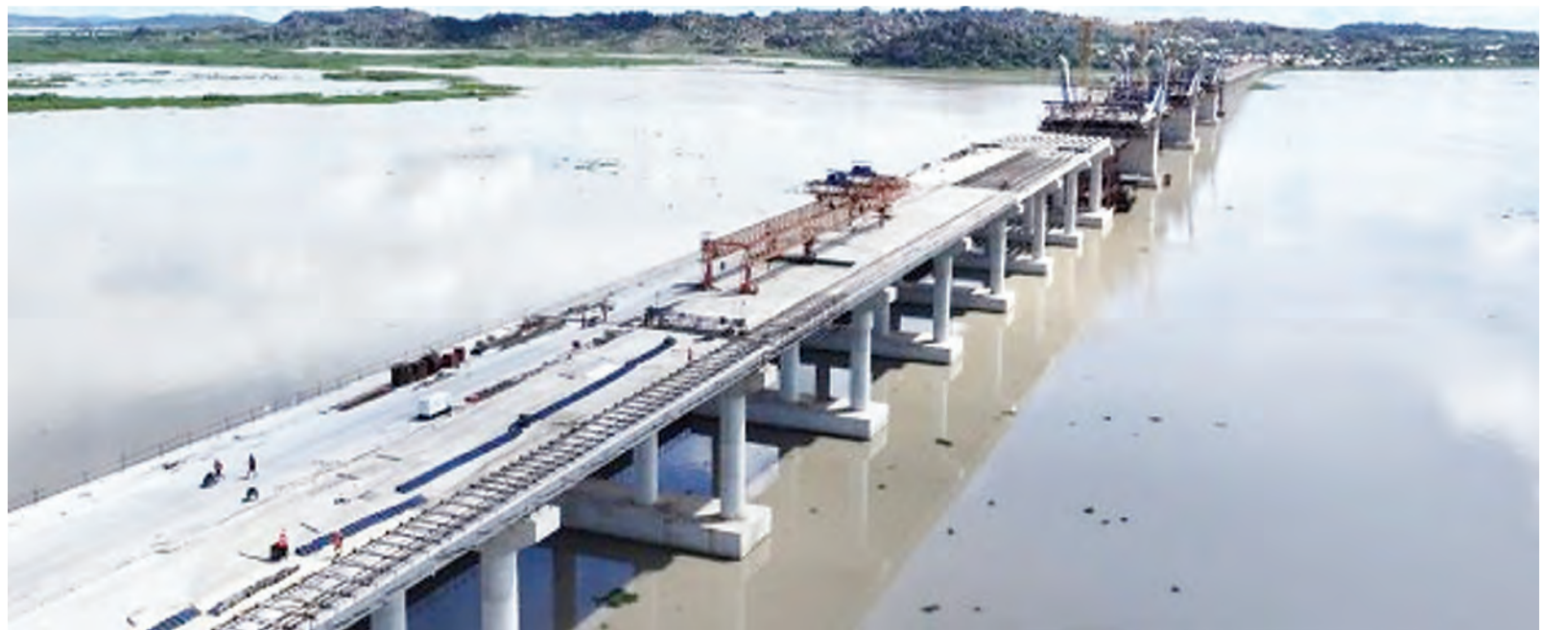
An aerial drone photo taken on April 11, 2024 shows the construction site of the Magufuli Bridge in Mwanza. Xinhua
