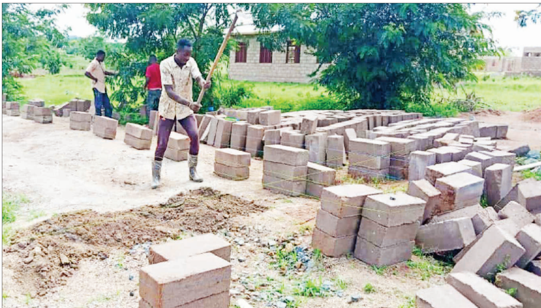
Preparations for the construction of classrooms for a secondary school at Kigera in Nyakatende ward in Musoma Rural constituency under way earlier this week. The school is expected to enroll students for Form One beginning next year. Photo: Guardian Correspondent
