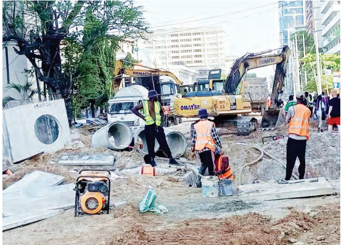
Implementation of Dar es Salaam's Bus Rapid Transit infrastructure development project in progress at the New Postal Office section in the heart of the city yesterday. Photo: Correspondent Jumanne Juma
