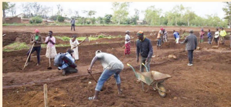
The file photo shows people constructing sports fields for refugees evacuated from Libya in the Gashora transit centre, eastern Rwanda, on Oct. 23, 2019.
