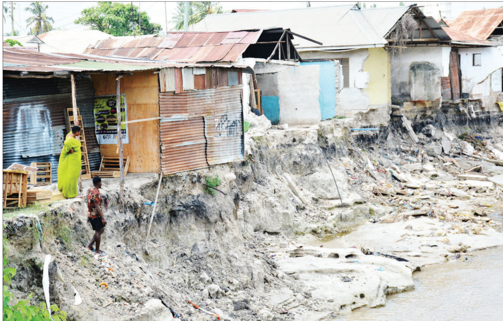
GOING, going almost gone. Mabibo resident Hemedi Abdallah (L) looks at their house at Mabibo in the outskirts of Dar es Salaam which is in bad shape following downpour along Msimbazi valley as captured yesterday. Photo: Correspondent Miraji Msala
