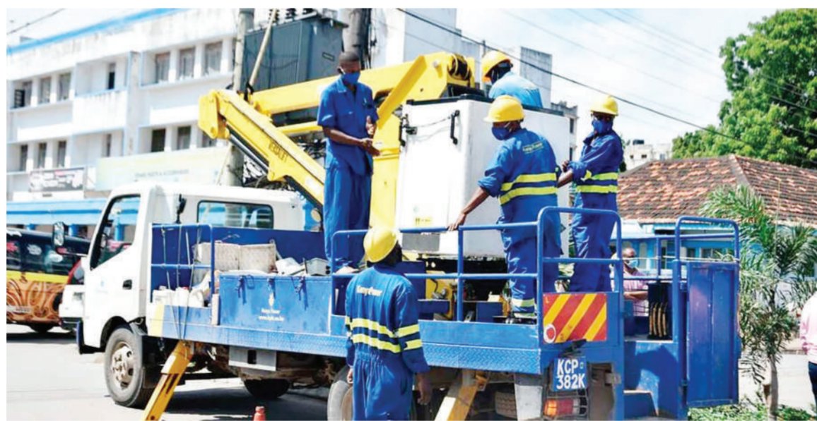
Kenya Power workers carry out repair works along Haile Selassie Road, Mombasa.
