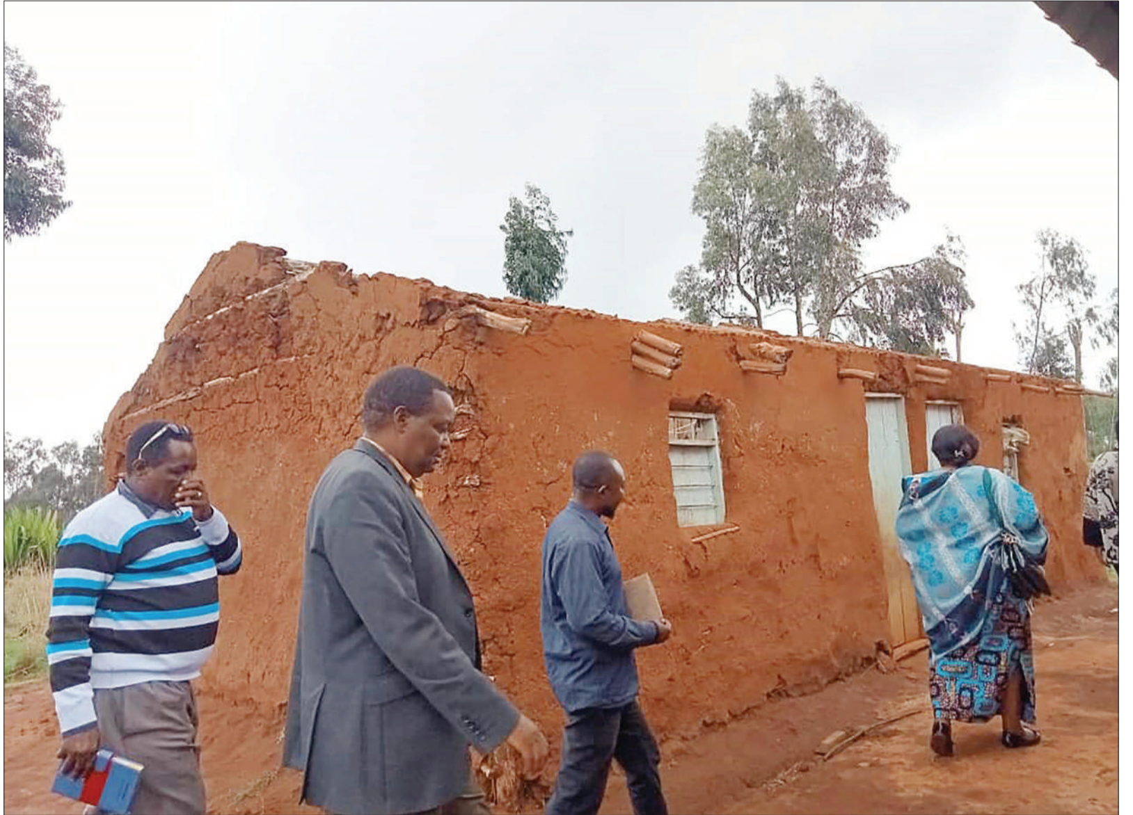
Babati Town Council chairman John Noya (2nd-L) and district executive director Anna Mbogo (2nd-R) on an inspection tour at the weekend of houses unroofed by strong winds at Kwankwari and Bashnet in Nar ward. Two Buma Hospital buildings were among those hit. Photo: Correspondent Gift Thadey
