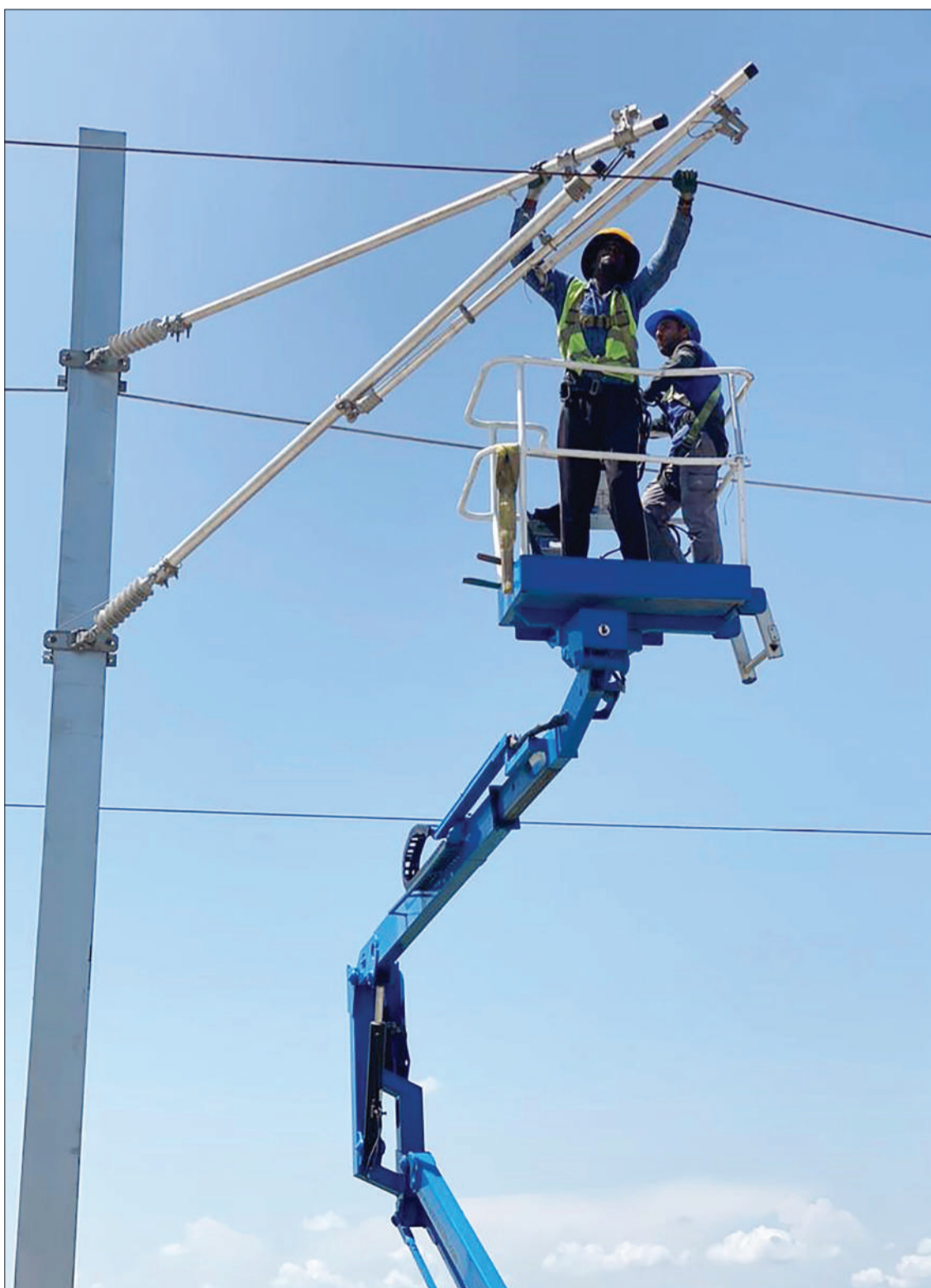
Technicians with Yapi Merkezi, an international contracting company specialising in rail engineering, design, manufacture and construction, pictured yesterday at work along the 165-km Isaka-Tabora stretch of the standard gauge railway project. Photo: Correspondent Shaban Njia
