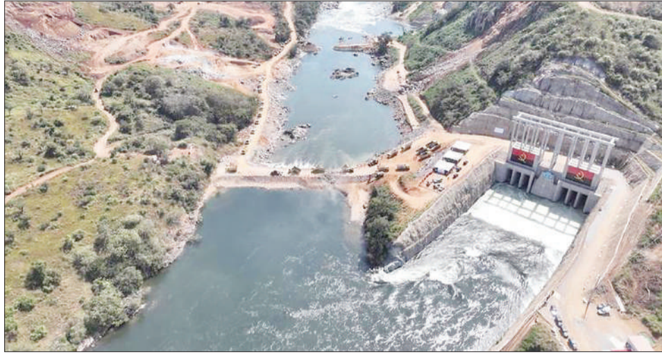
This aerial photo taken on May 20, 2023 shows a ceremony for the temporary diversion of the Cuanza River at the site of the Chinese-built Cacufo-Cabaca Hydropower Station in Cuanza Norte province, Angola. XINHUA
