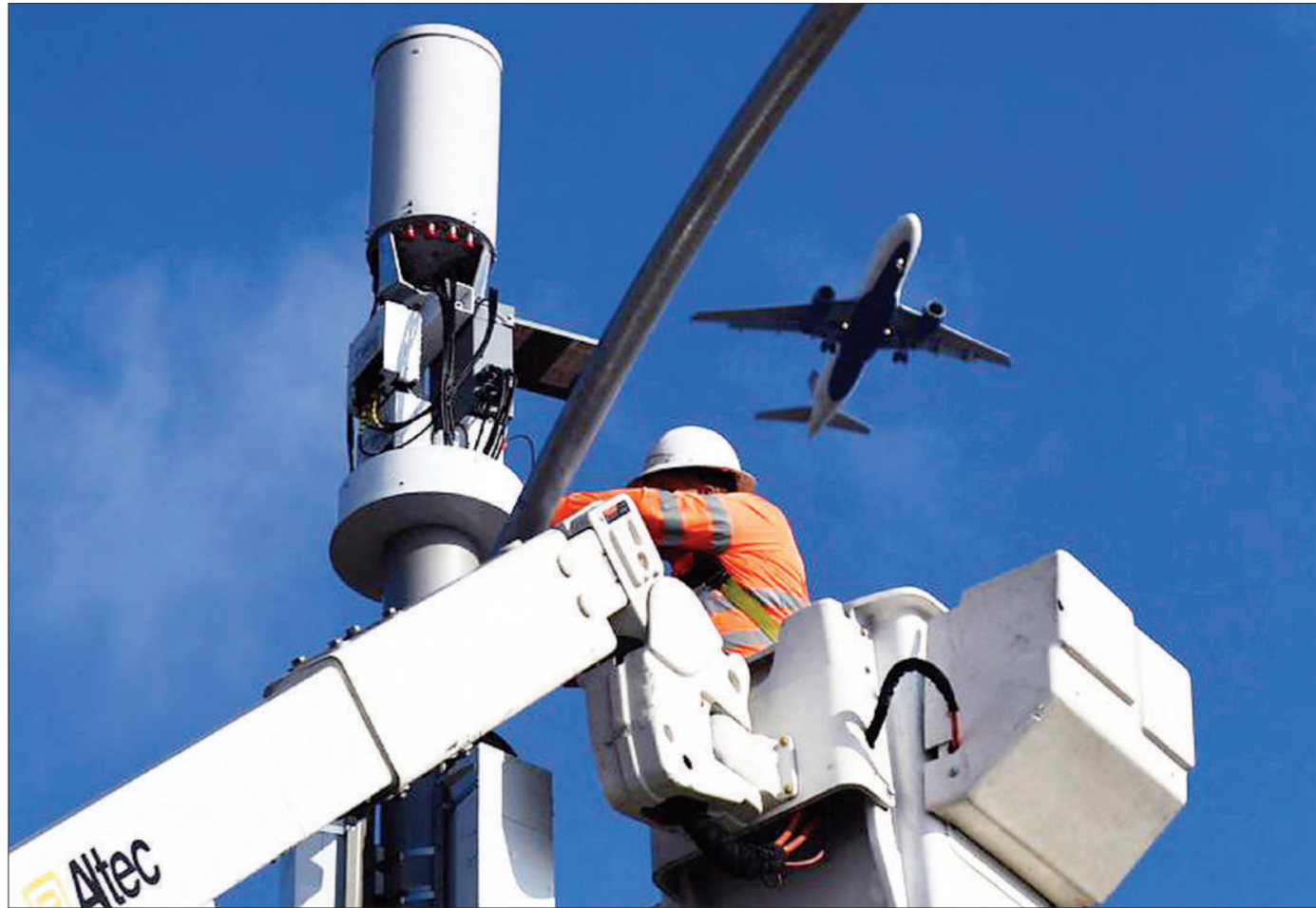
A worker installs 5G cellular equipment on a light pole as an Airbus A320 airplane lands at Los Angeles International Airport on Jan 19. File photo
