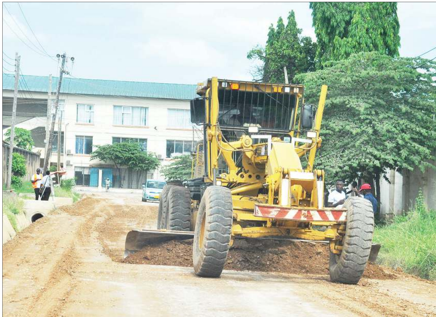
A grader levels Dar es Salaam's Sewa Road, which was rehabilitated only months ago but is already pot-holed, as spotted yesterday just next to the offices of The Guardian Limited and ITV/Radio One in the city's Mikochei Light Industrial Area. Photo: John Badi
