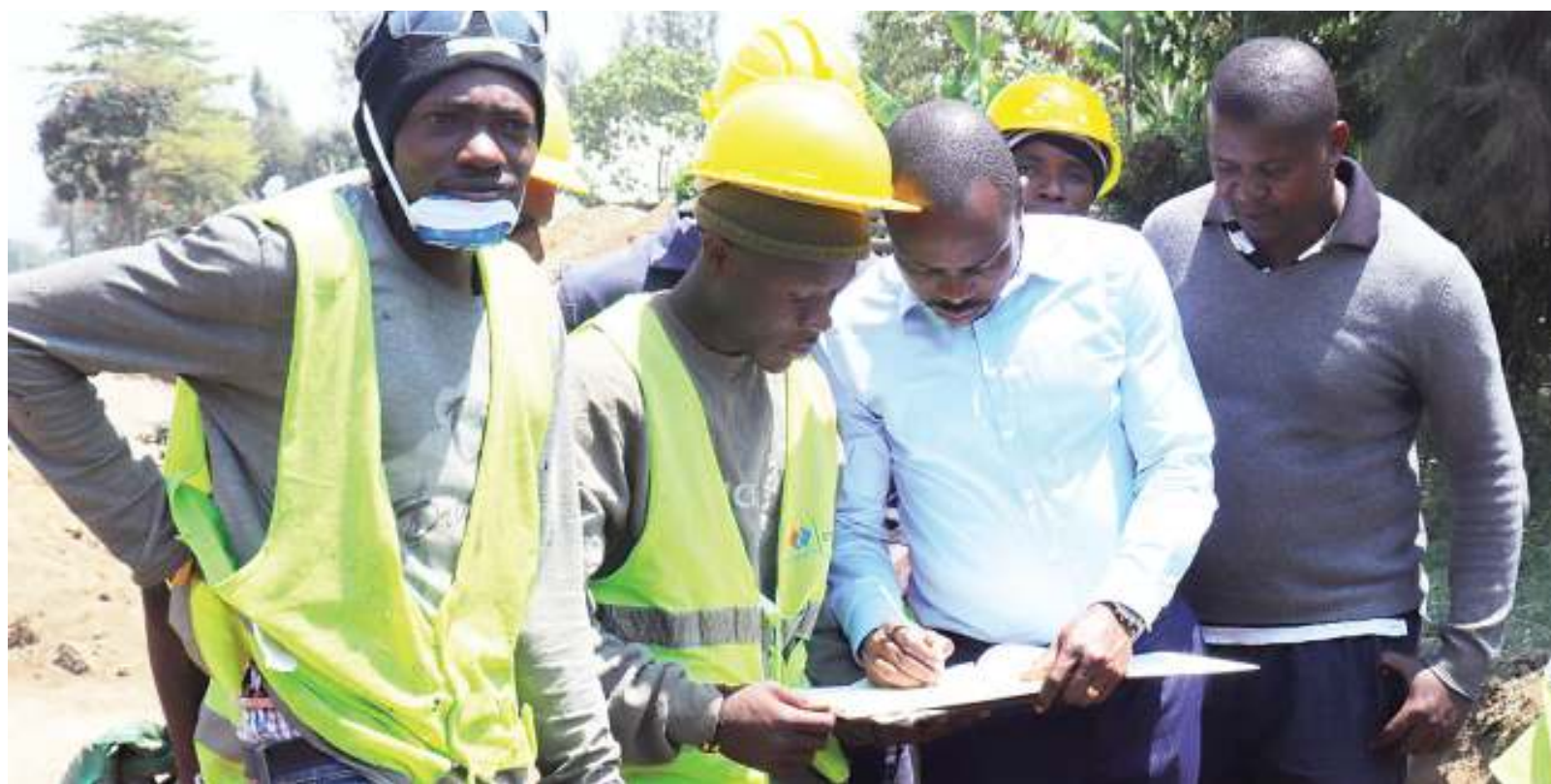
Arumeru district commissioner Jerry Muro (2nd-R) registers in a visitors' book at the site of a water project he toured yesterday to assess the progress contractors had made in implementing it. Photo: Correspondent Woinde Shizza
