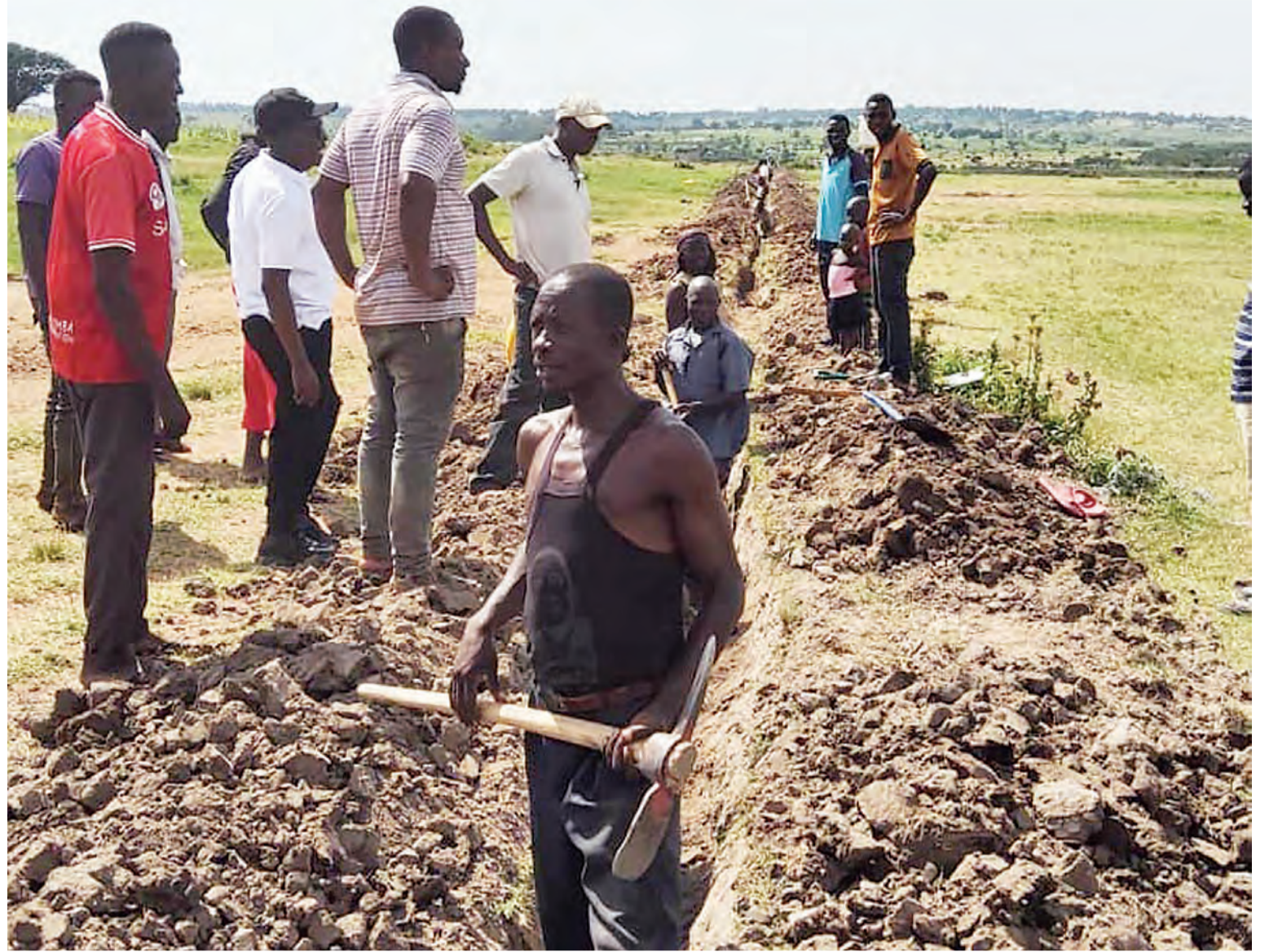
Musoma Rural legislator Prof Sospeter Muhongo (2nd-L, in white T-shirt) pictured on Wednesday witnessing the digging of a trench in Tegeruka ward in which to lay pipes in implementation of a project meant to pump water from Lake Victoria through Tegeruka and Mugango wards to Butiama District. Photo: Guardian Correspondent
