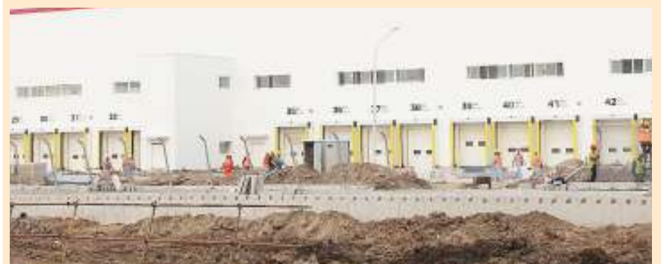
Workers are seen at the construction site of US electric car maker Tesla's Gigafactory in Shanghai.
