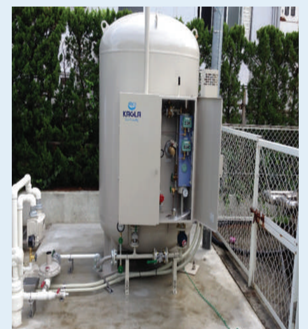
Kagla Vaportech Corp's Integrated LP Gas Supply System would contribute to Clean Cooking.
