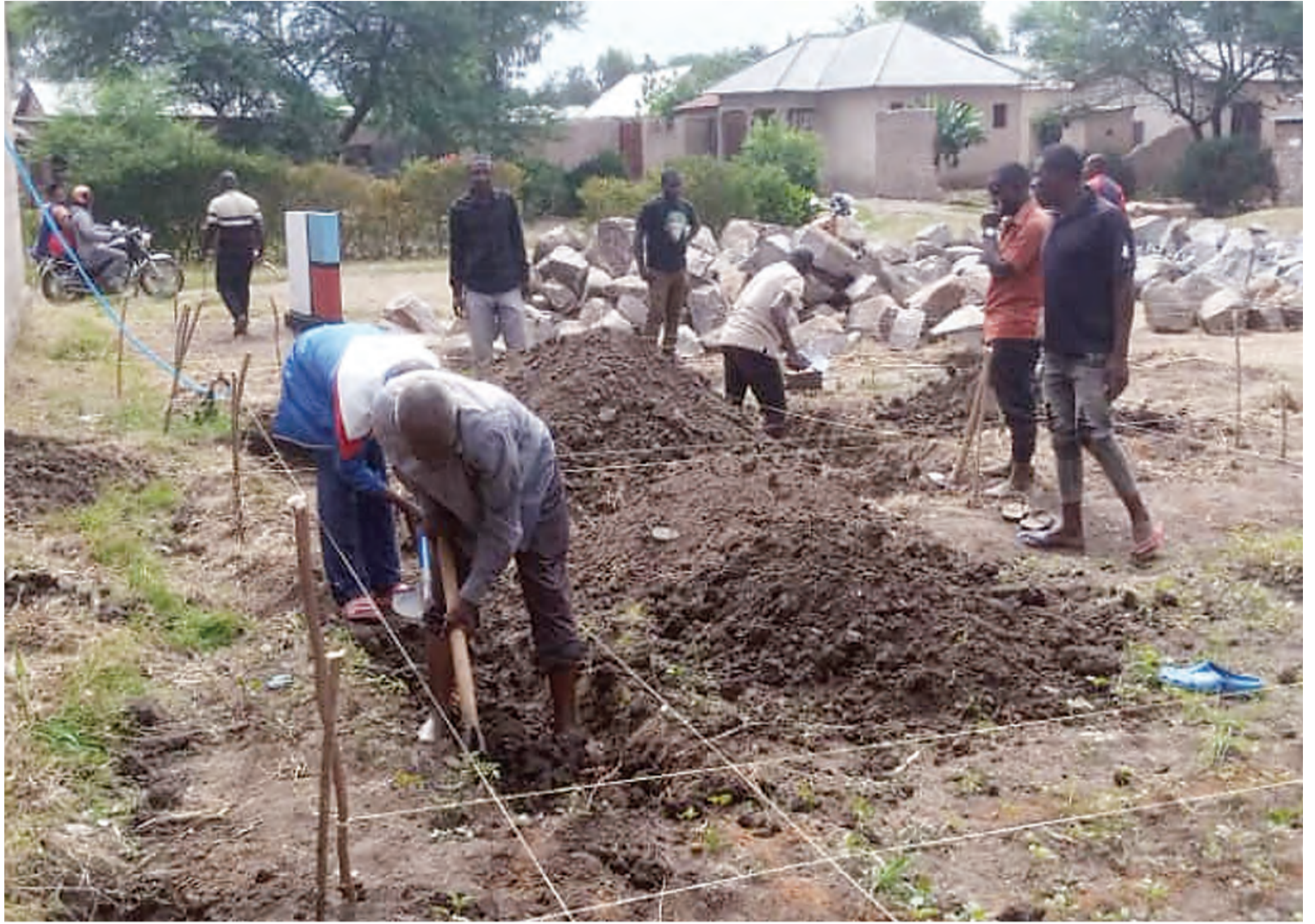
Preparations for the construction of the opposition Chadema's Musoma Urban district office in progress at Nyakato in Musoma municipality yesterday. Photo: Guardian Correspondent
