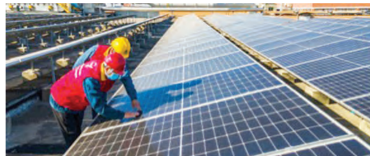
Employees of the Jindong power supply company under the State Grid maintains photovoltaic panels on the roof of a workshop in a factory in Jindong district, Jinhua, east China's Zhejiang province, Dec. 15, 2022. (Photo by Hu Xiaofei/People's Daily Online)
