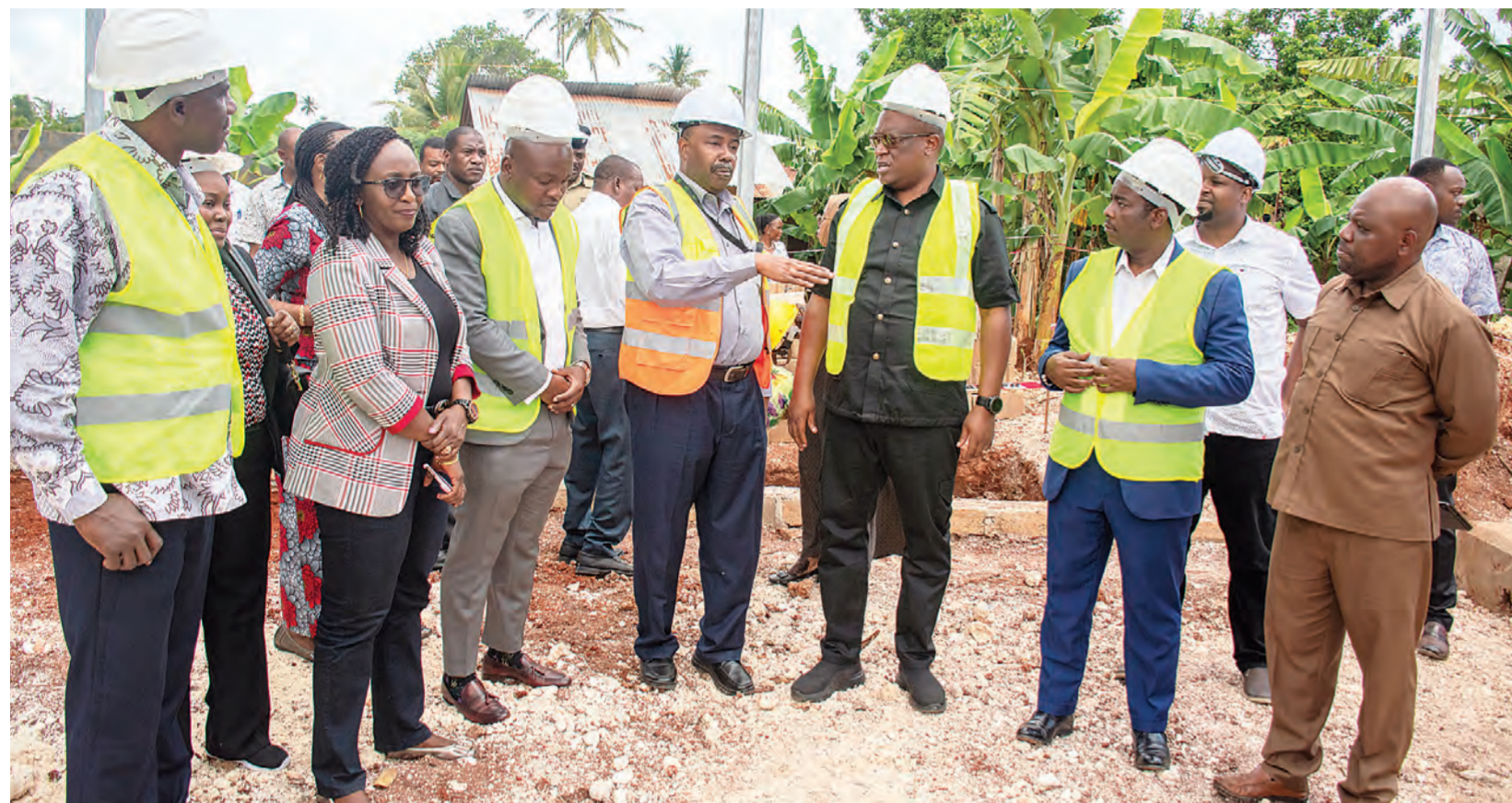
Zantel project manager Mohamed Ahmed Jai (gesturing) briefs Information, Communications and Information Technology minister Nape Nnauye (to his left), who was on an inspection tour of the construction of Tigo-Zantel communication towers in Zanzibar on Monday. Photo: Guardian Correspondent
