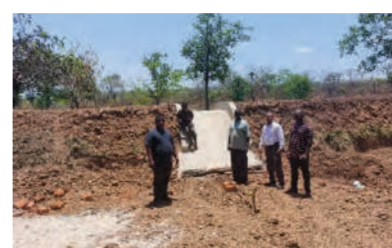
Photo: Overflow (Spillway) of the Rain Water Harvesting Reservoir Project number: N5 from the list of demonstration projects
