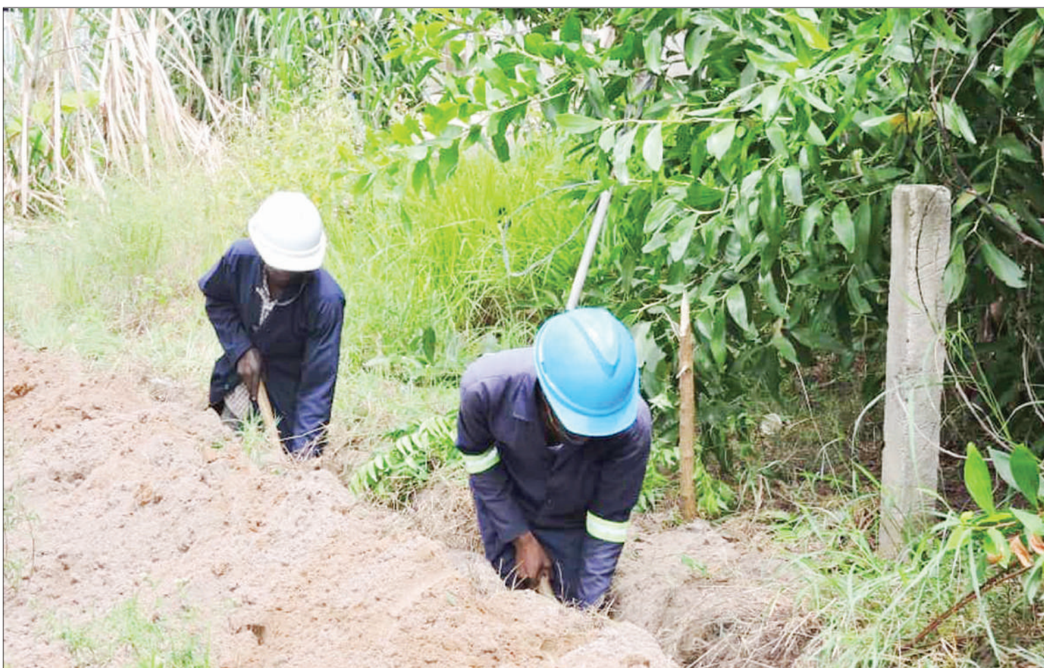
Dar es Salaam Water and Sanitation technicians dig a trench at Minondo in Kigamboni District at the weekend to enable the laying of a 150-meter pipe. Photo: Guardian Correspondent
