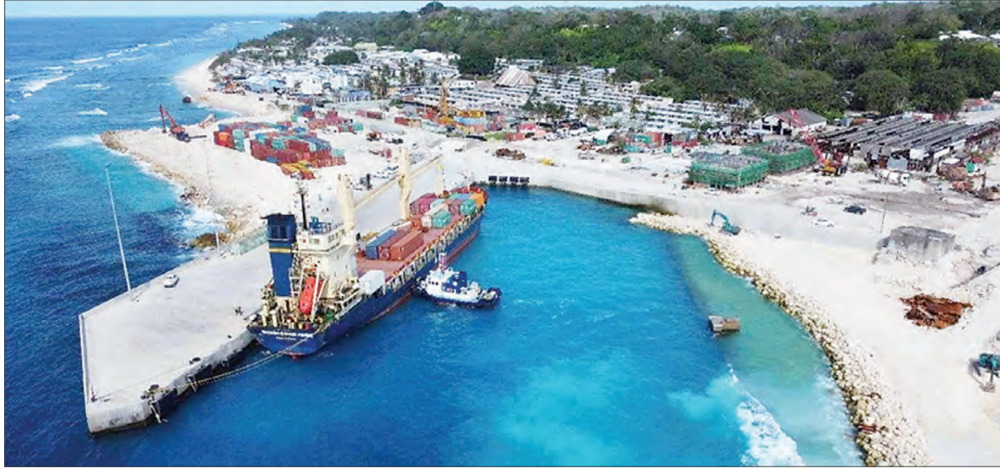
Photo shows the upgrading and renovation project of Awo Port Terminal in Nauru undertaken by a Chinese enterprise. [Photo/Li Lingfeng]
