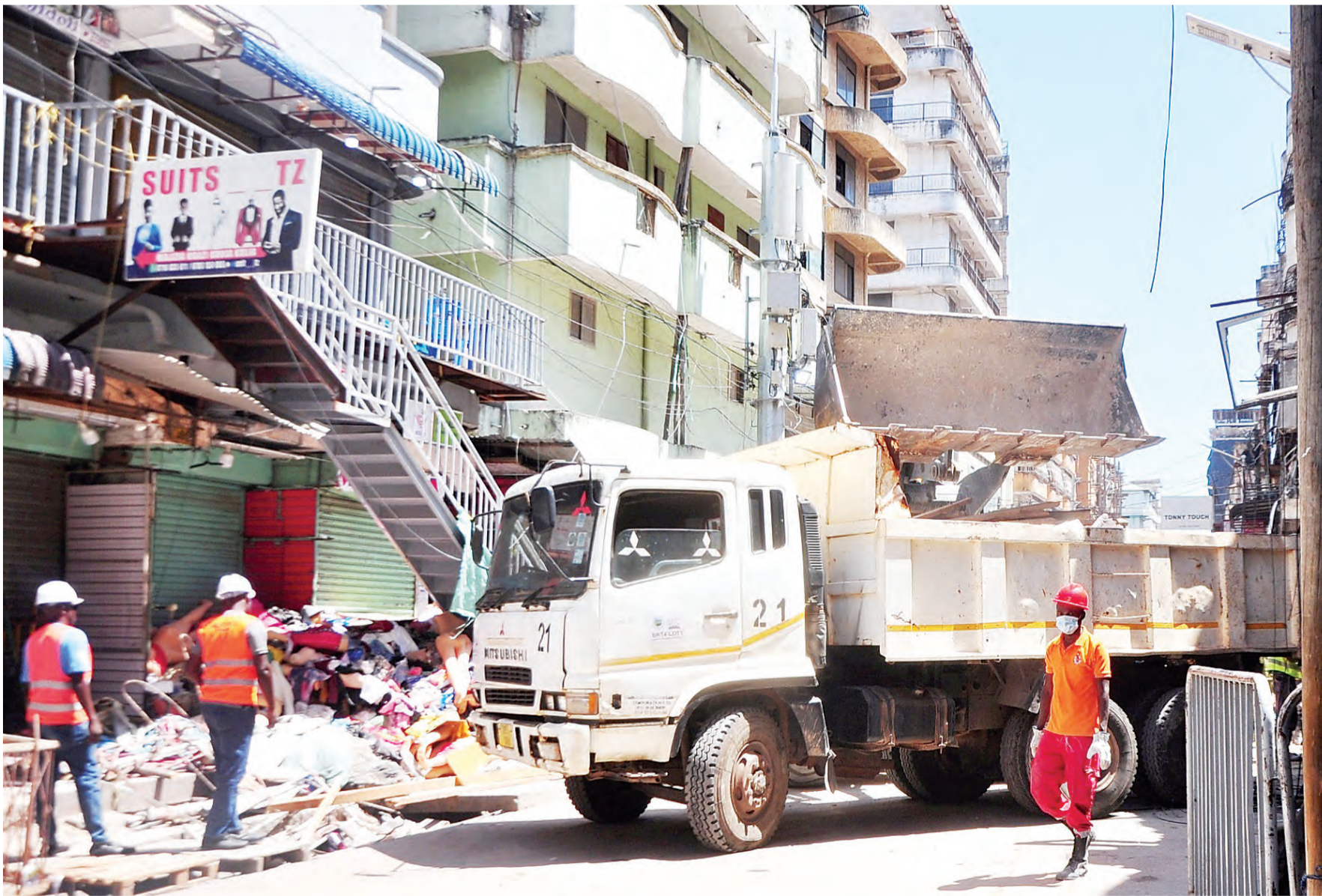
Clearing of rubble continues yesterday at the site of the multi-floor building which collapsed in Dar es Salaam's sprawling Kariakoo market zone on Saturday, leaving several people dead and dozens injured. Photo: Correspondent Imani Nathaniel
