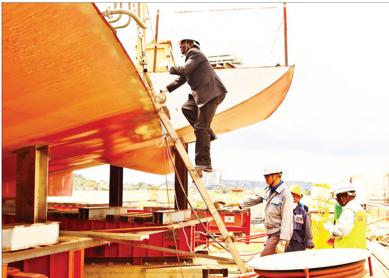
Works and Transportation minister Dr Leonard Chamuripo pictured in Mwanza city yesterday climbing a ladder aboard the state-of-the-art US$39 million MV Mwanza 'Hapa Kazi Tu'. The ship is being built at the Mwanza shipyard by Gas Entec, a South Korean engineering and design firm with shipbuilding experience. Sources say the vessel's capacity will be 1,200 passengers and 400 tonnes of cargo alongside 20 small vehicles and three trucks, this qualifying it as the largest in Africa's Great Lakes region. Photo: Guardian Correspondent
