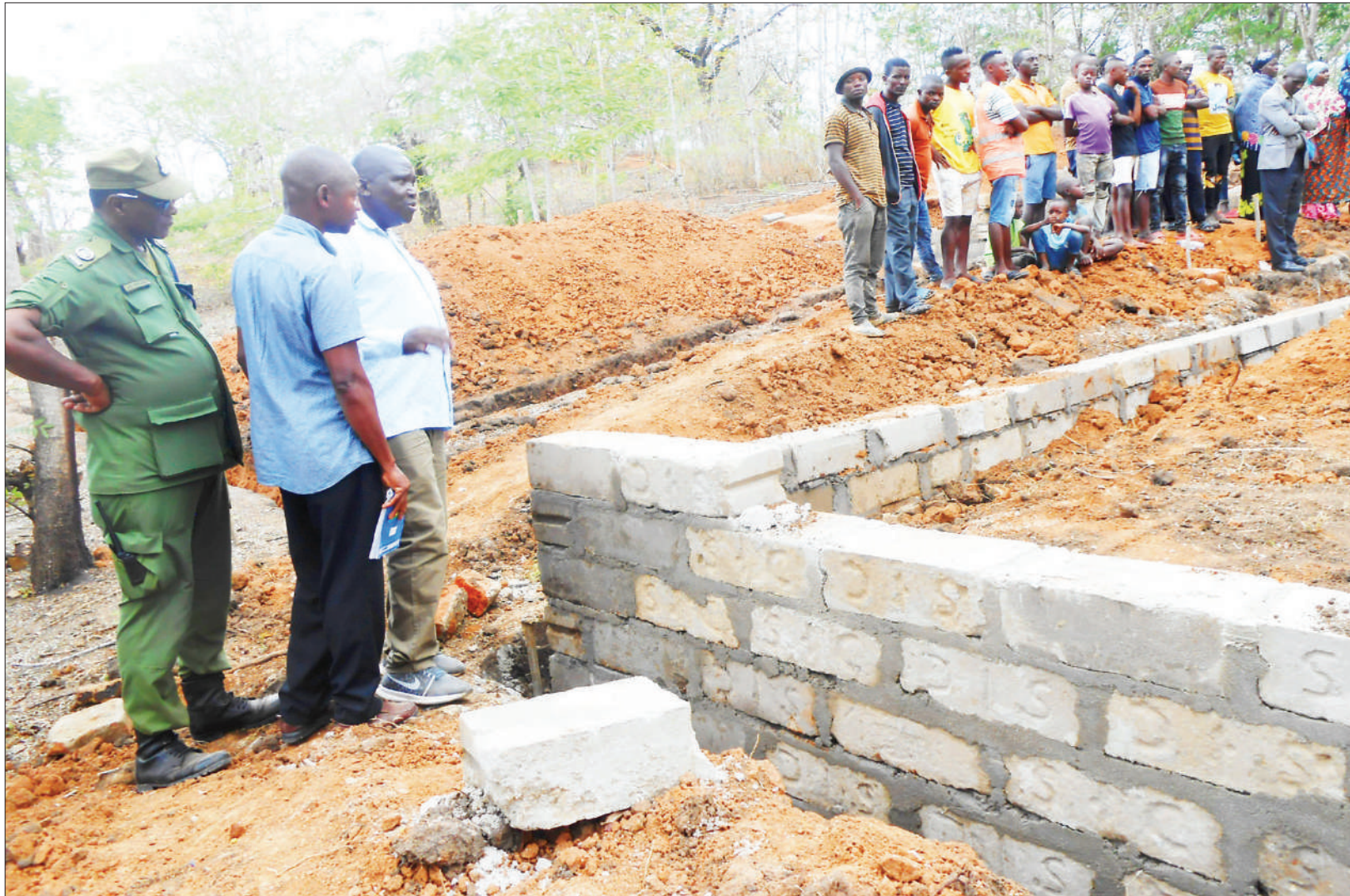
Kilindi district commissioner Abel Busalama (3rd-L) assesses progress in the construction of classrooms and teachers' office at Kimbe Secondary School on Wednesday. Photo: Correspondent Dege Masoli
