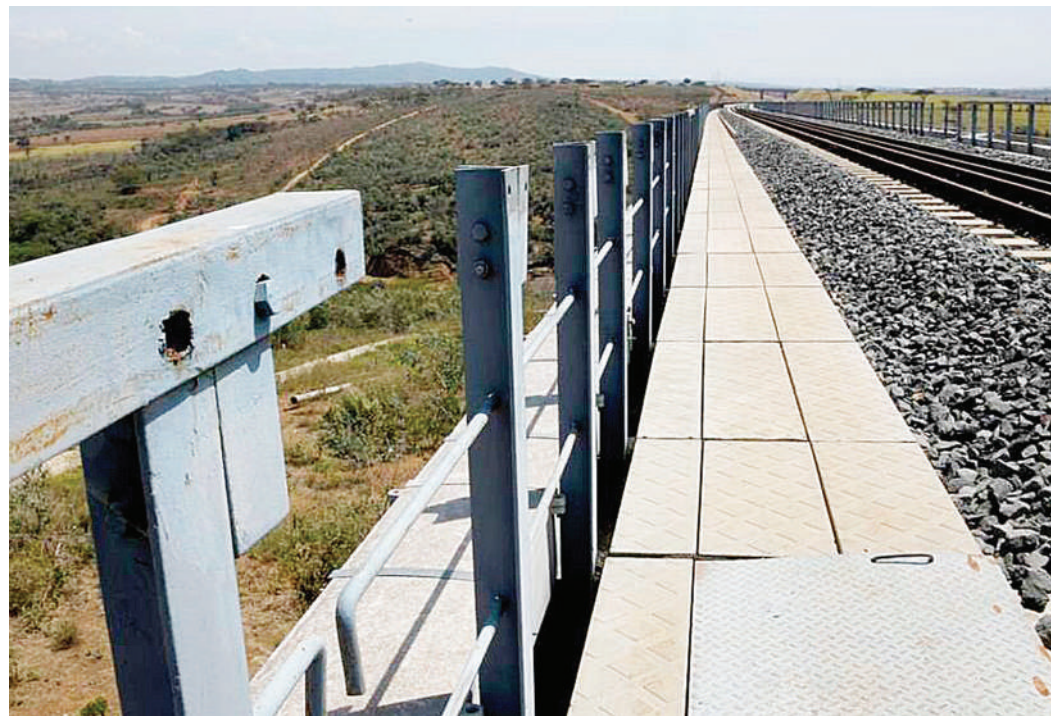
The vandalised SGR in Murtoto, Suswa.
