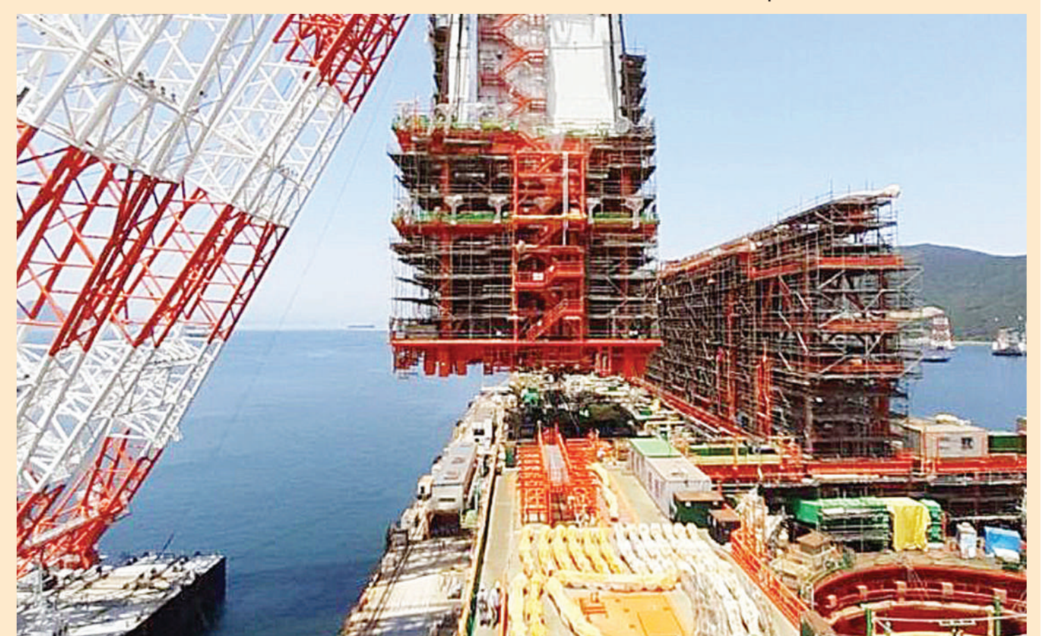
A floating platform to be used in the production of Liquefied Natural Gas (LNG) in the Coral South gas field being offloaded off the coast of Cabo Delgado.
