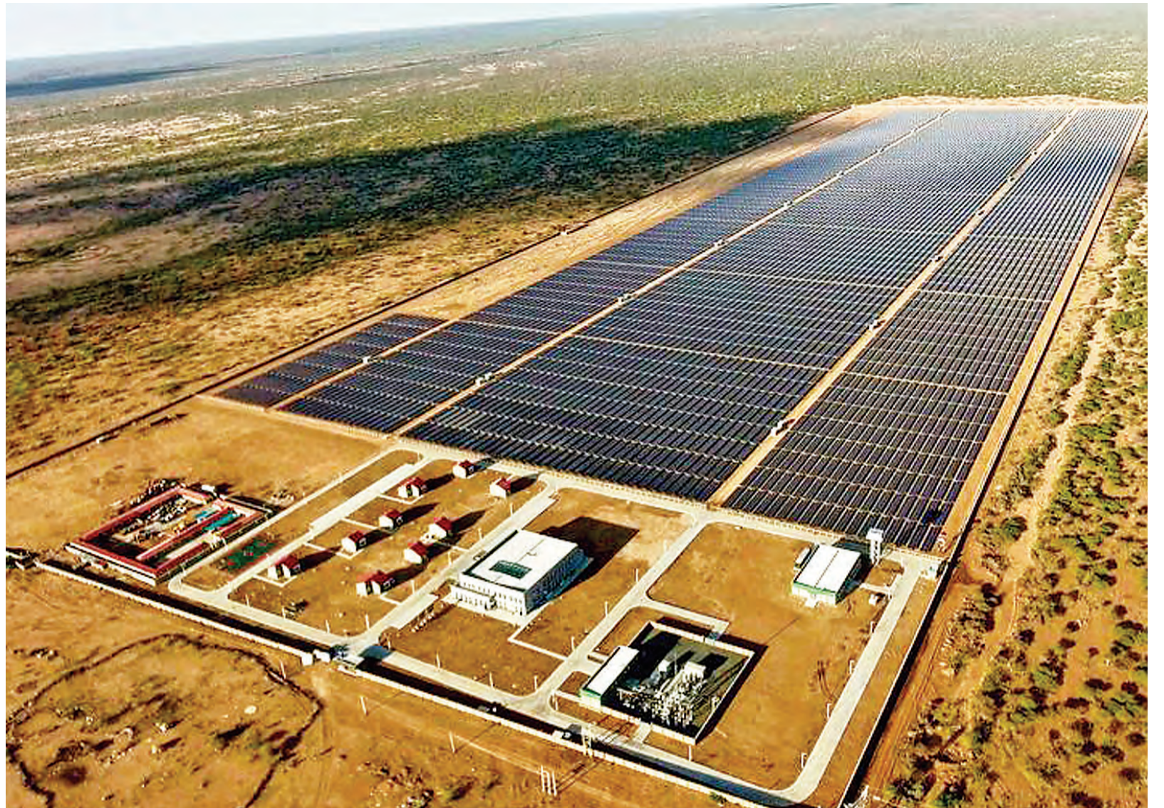
Garissa Solar Power Plant in northeastern Kenya.
