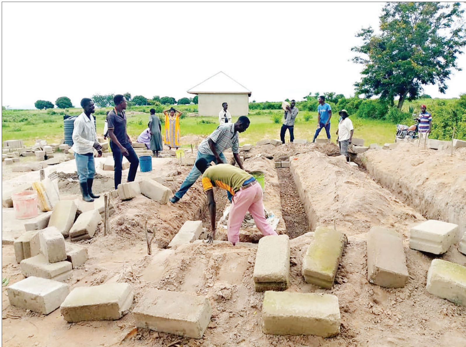
Masons build classrooms foundation at Muhoji secondary school located at Muhoji village in Musoma Rural District, Mara Region which is expected to be opened next year. Photo: Guardian Correspondent
