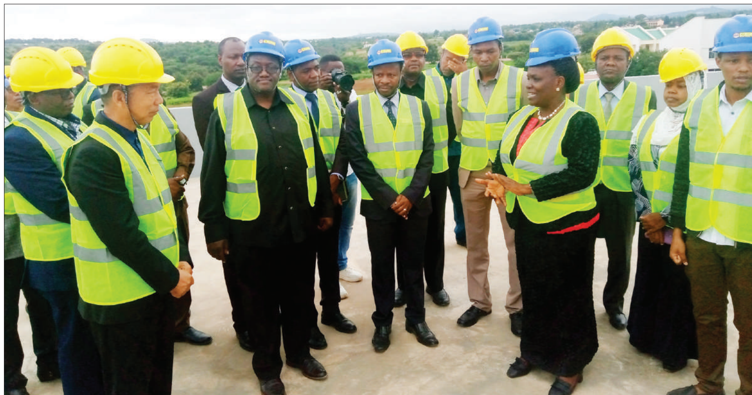
Joyce Ndalichako Minister for Education, Science and Technology (4th R) gives directives to Tanzania Atomic Energy Commission management and Board of Directors during her visit to inspect the construction of a new laboratory building in Arusha yesterday. Photo: Correspondent Daniel Sabuni
