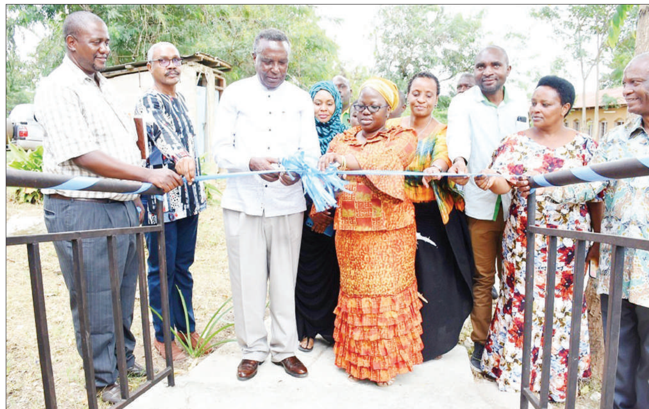
Bagamoyo district commissioner Zainab Kawawa (in headscarf and glasses) and Hassan Maajar Trust HMT vice chairman Shariff Hassan Maajar (3rd-L) cut a ribbon when handing over toilet facilities and supplies donated under the trust's 'Quality Toilets in All Schools' project to Bagamoyo's Nia Njema and Majengo primary schools at the weekend. Photo: Guardian Correspondent
