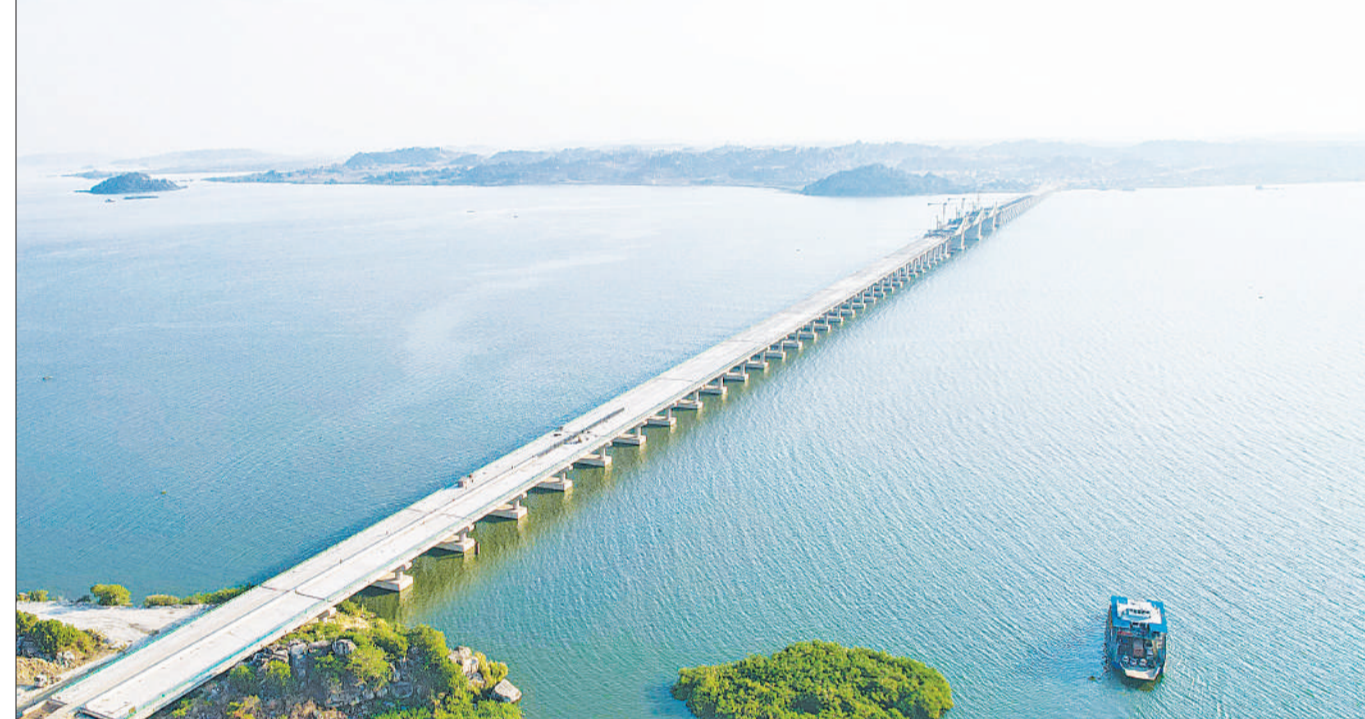
This is a view of J. P. Magfuli Bridge, now 90 per cent done, as captured by the Works ministry only days ago. It is 3.2 kilometres long and easily one of the major infrastructure projects being implemented by the government. It runs through Lake Victoria waters, as a crucial link on the Usagara-Sengerema-Geita highway. It is widely expected to be instrumental in vastly improving transportation across all regions in Tanzania's Lake Victoria zone. This will be chiefly by significantly enhancing the movement of goods and people between these regions and other parts of the country. Photo courtesy of Works ministry
